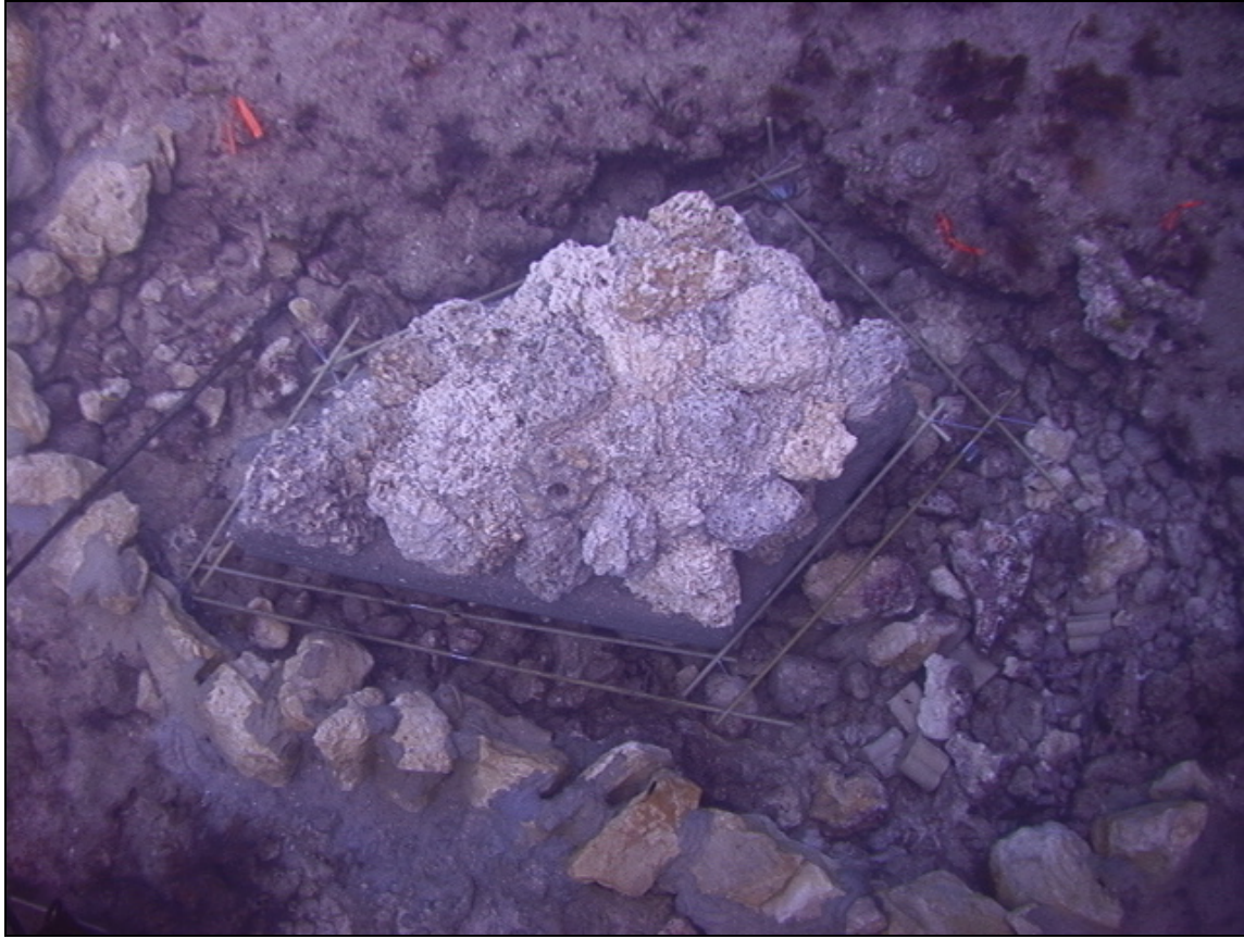
Figure 8. Reef restoration module and reinforcing rods in excavation crater ready to accept tremie pour concrete (photo credit: FKNMS).
