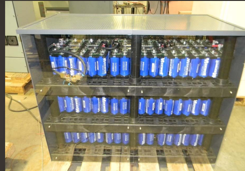
Maxwell super capacitor bank
