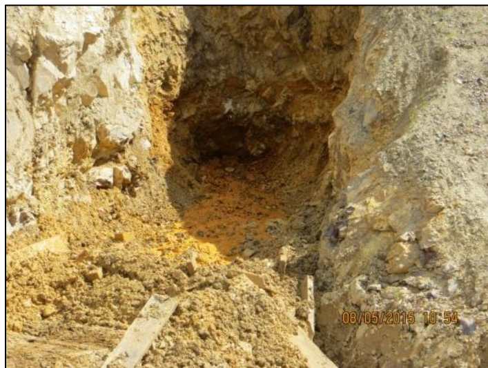
The flow of water escaping from the adit has increased and turned orange. Wood planks, placed to direct water towards the channel on the right side of the adit, are also visible. Source: EPA.
