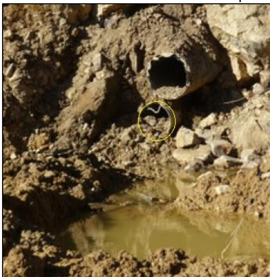
The drainage pipe, highlighted in yellow, is revealed during EPA’s 2014 excavation of the adit. Water is pooling on the waste rock dump surface, just below the drainage pipe. Source: Environmental Restoration.
