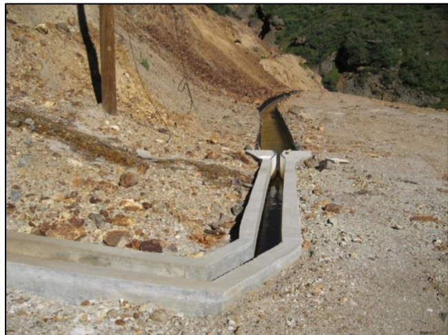
The concrete channel installed by DRMS in 2009. Source: Environmental Restoration.
