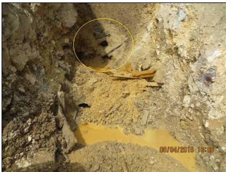
In this photo from 4:08 p.m. on August 4, the EPA crew has unearthed the plug (highlighted in yellow). The end of a section of pipe is visible in the mound in front of the plug. Source: EPA.
