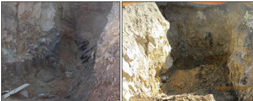
On morning of August 5, 2015, the plug is still visible (left). Shortly thereafter, it was buried with backfill (right). Source: Environmental Restoration/EPA.
