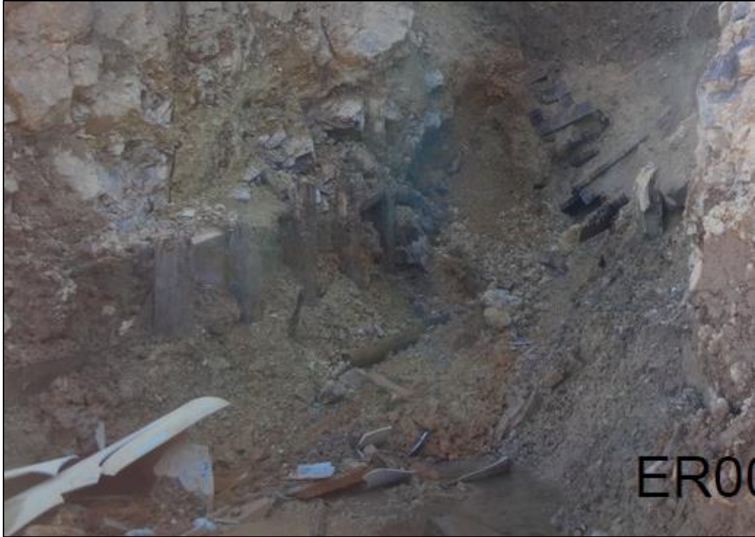
Shards of the removed drainage pipe (lower left) in front of the excavated adit. Source: Environmental Restoration.
