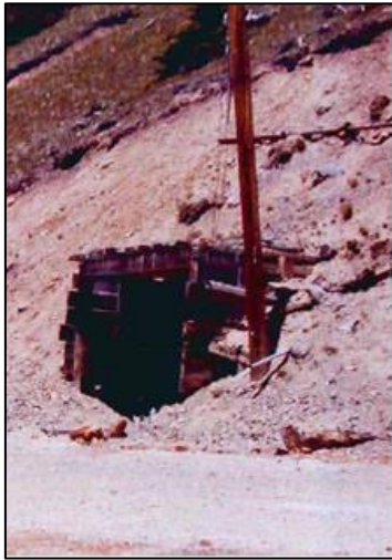
The portal structure, prior to DRMS's work. Source: DRMS.
