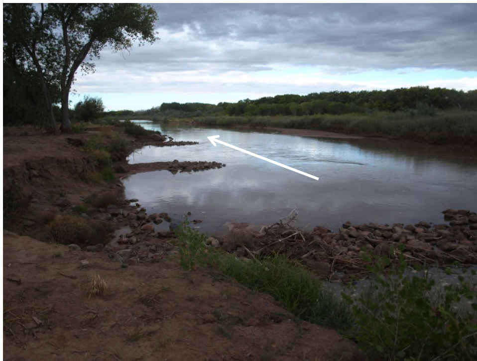
Photo 12: Bank erosion at Santa Ana RM 205.8 (AuBuchon, October 2015)
