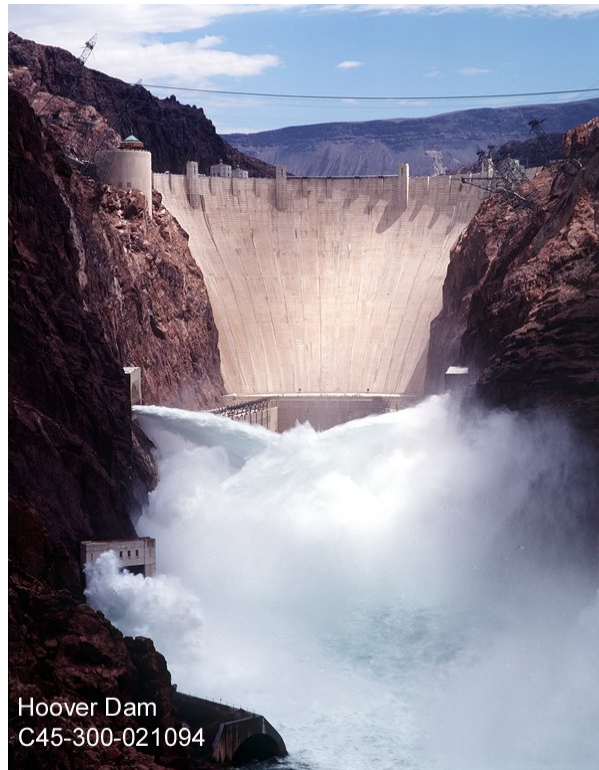
Figure 3 - Hoover Dam downstream releases.
