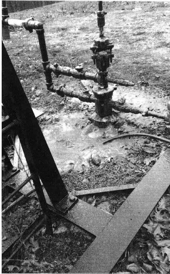
Contamination caused by an oil and gas well failure. ©FracTracker Alliance
