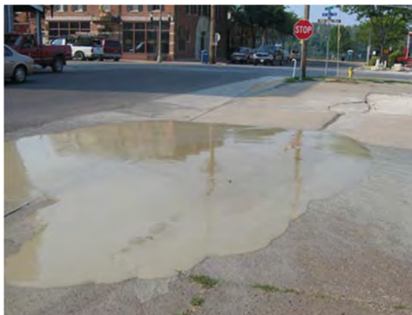
Figure 4: Inadvertent drilling fluid return surfacing through cracks in pavement
