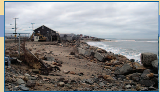
Increasing sea levels and more intense storms will impact our shores. This rocky barricade, or revetment, was scattered by an intense storm that caused sea water to overtop the rocks.
