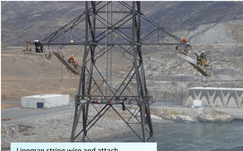
Lineman string wire and attach hardware on special 316 foot tall river crossing tower for Grand Coulee cable replacement project.
