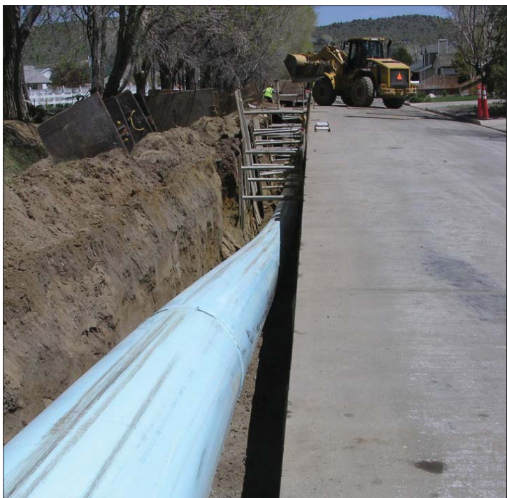
Michelle Stamates, Nevada Division of Environmental Protection Installation of 450 linear feet of 24-inch fusible PVC below existing utilities in Carson City, NV.
