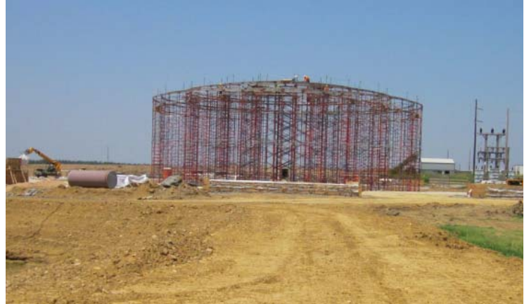
Oklahoma Department of Environmental Quality Clearwell at the Broken Arrow Municipal Authority in Oklahoma.
