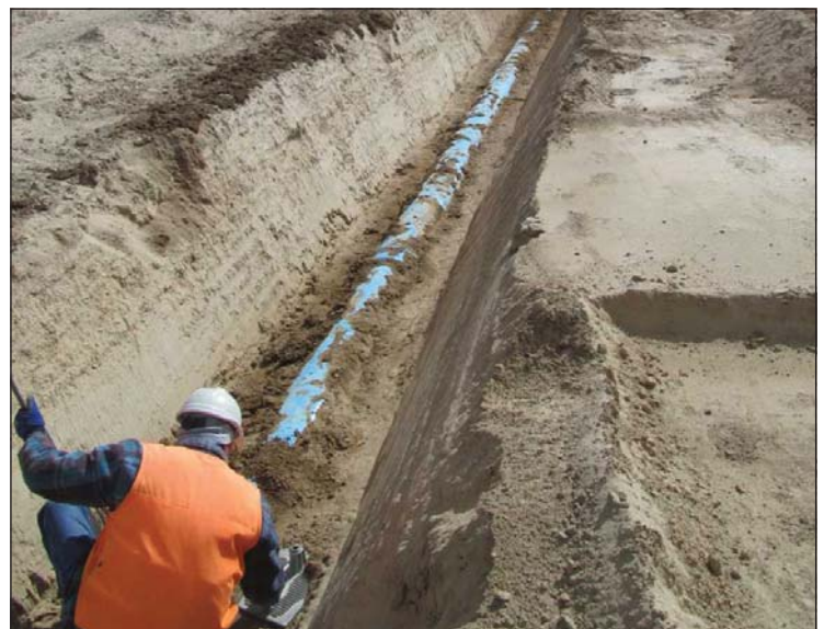
Gordon Cole, Shaw Engineering Installation of more than 35,000 linear feet of new 14-in PVC transmission line in Tonopah, NV.
