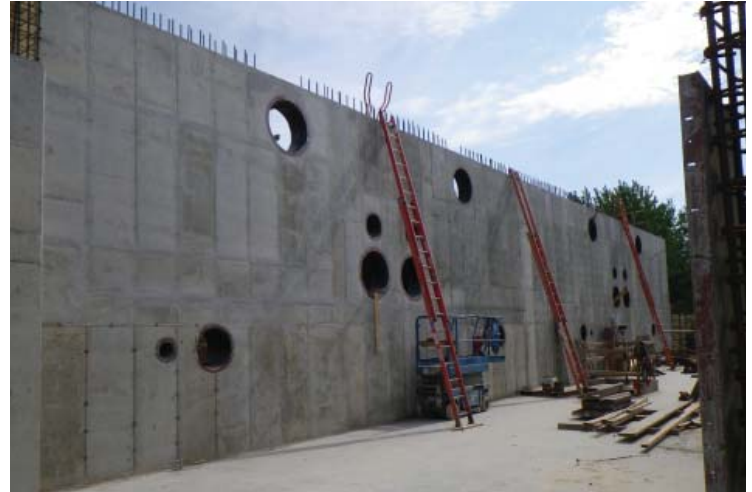
Chad Kolstad, Minnesota Department of Public Health New surface water treatment plant in Fairmont, MN. The current plant was constructed in 1926 and needed to be replaced. The new plant will have biologically active GAC filters to help with taste and odor complaints.
