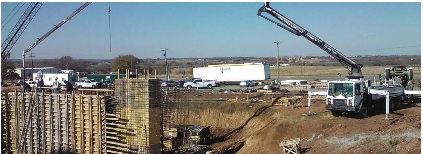
Super Pulsator Water Treatment Plant at the Davis Municipal Authority in Oklahoma.
