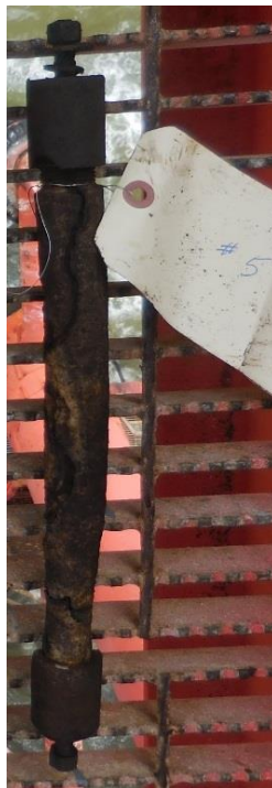
Figure 27 - Insulated Hanger #5 with arcing evident (April 27, 2015)
