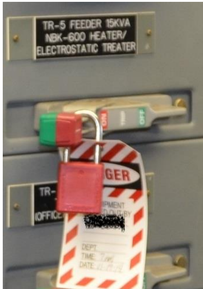
Figure 13 - Heater treater breaker in MCC Building, as observed by BSEE Investigators on November 21, 2014 (Name Redacted by BSEE)
