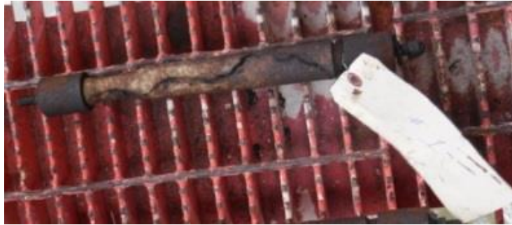
Figure 26 - Insulated Hanger #1 with arcing evident (April 27, 2015)
