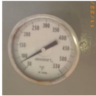
Figure 17 - Temperature Gauge on Transformer (November 22, 2014)
