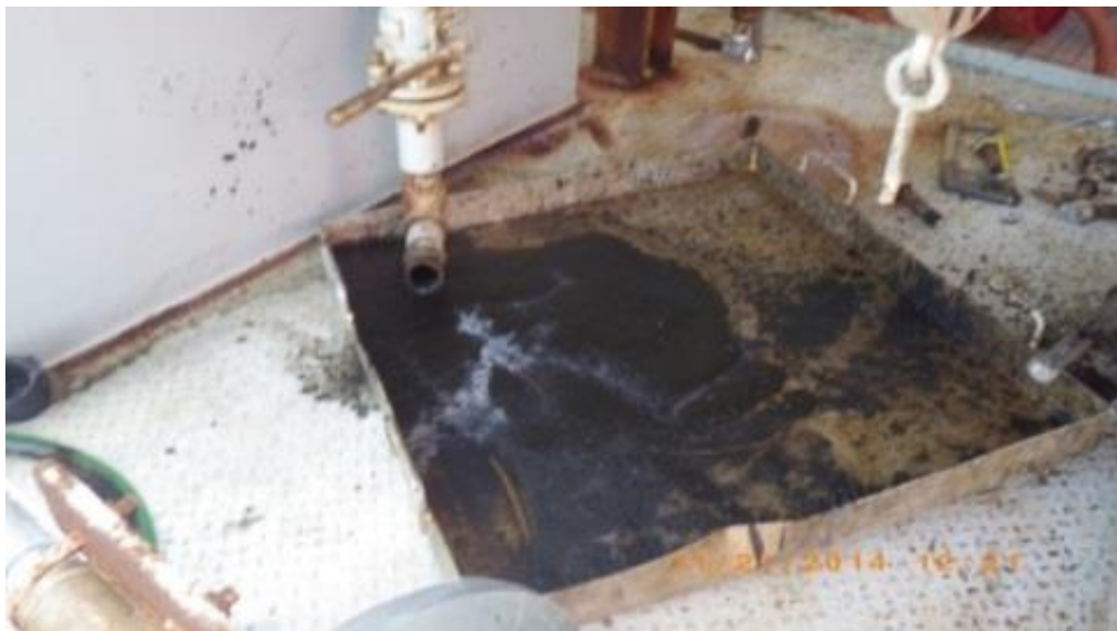
Figure 7 - Skid/Drip Pan Below Heater Treater Manway Hatch (November 21, 2014)
