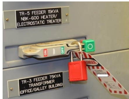
Figure 20 - Heater treater breaker 'Off' (November 21, 2014) (Name Redacted by BSEE)
