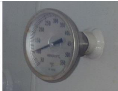
Figure 16 - Temperature Gauge on Transformer (November 21, 2014)
