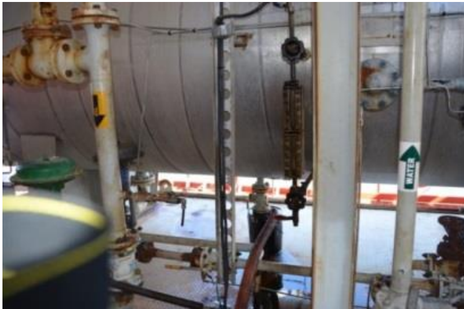
Figure 8 - Drainage Bucket Under Heater Treater (November 21, 2014)
