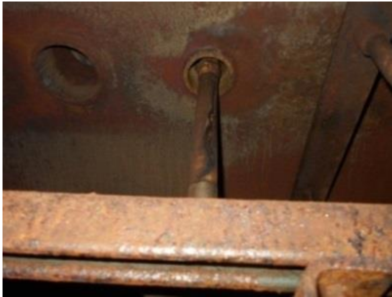
Figure 25 - Internal View of High Voltage Entrance Bushing (April 25, 2015)
