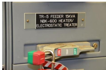
Figure 19 - Heater treater breaker 'On' (November 21, 2014)
