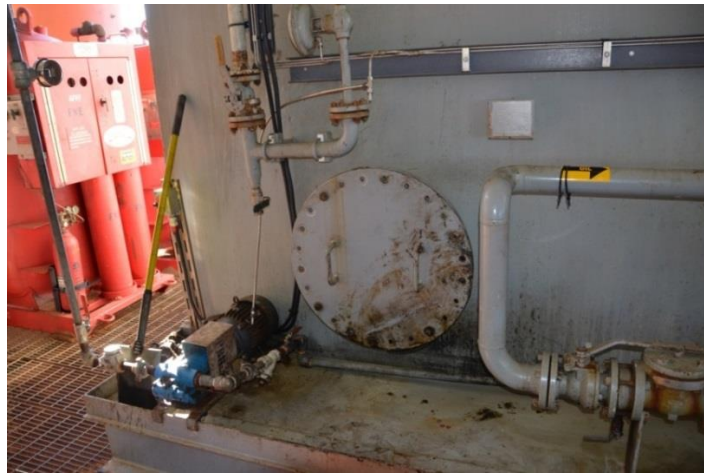
Figure 6 - Dry Oil Tank Hatch (November 21, 2014)
