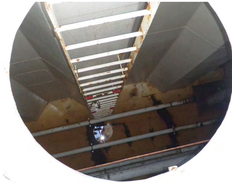
Figure 8. A holding tank, empty
