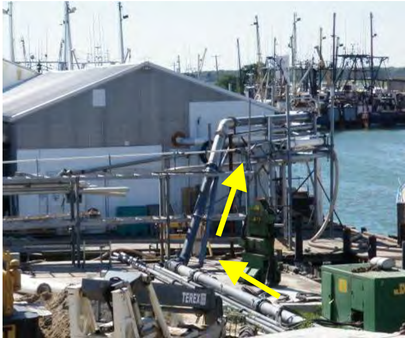
Figure 24. Transportation pipes and hoses entering the processing facility after coming from the dock.
