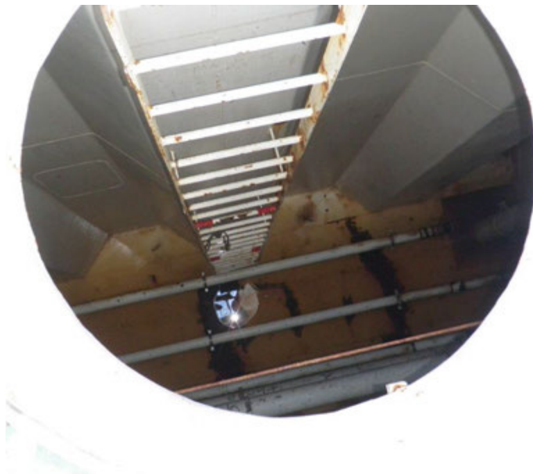
Figure 8. A holding tank, empty
