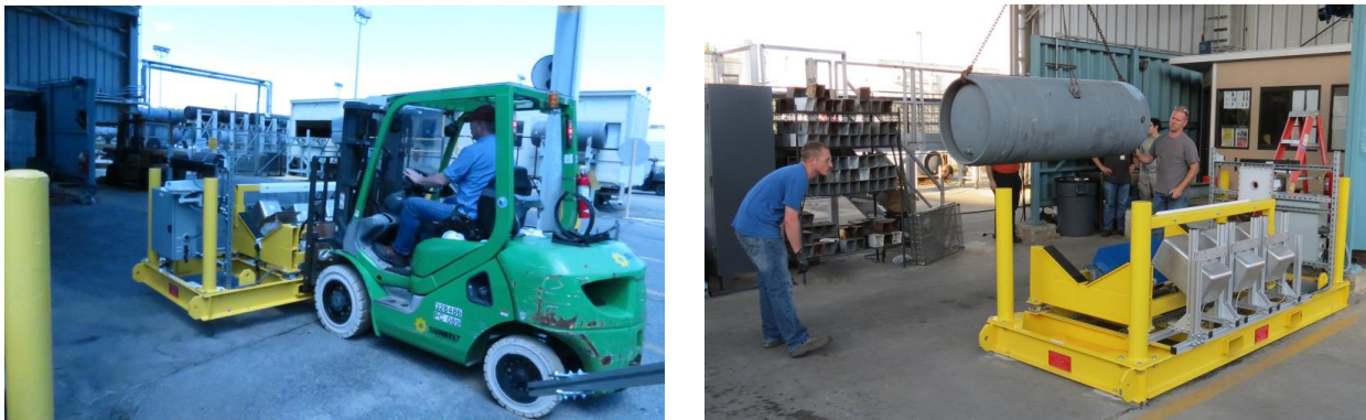
Figure 37. Forklift placement of the platform at the deployment location (left); placement of first cylinder on the UCVS prototype platform using the overhead crane (right).
