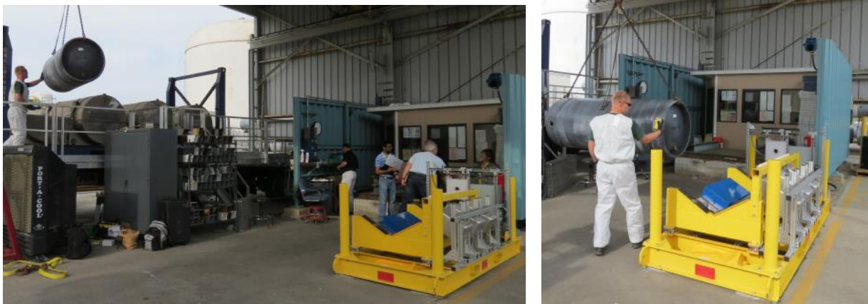
Figure 39. Retrieve a full cylinder from overpack (or other on-site location) and place cylinder on the UCVS platform using the overhead crane. For a typical cylinder scan, the valve/nameplate end of the cylinder should be facing the scale shack.
