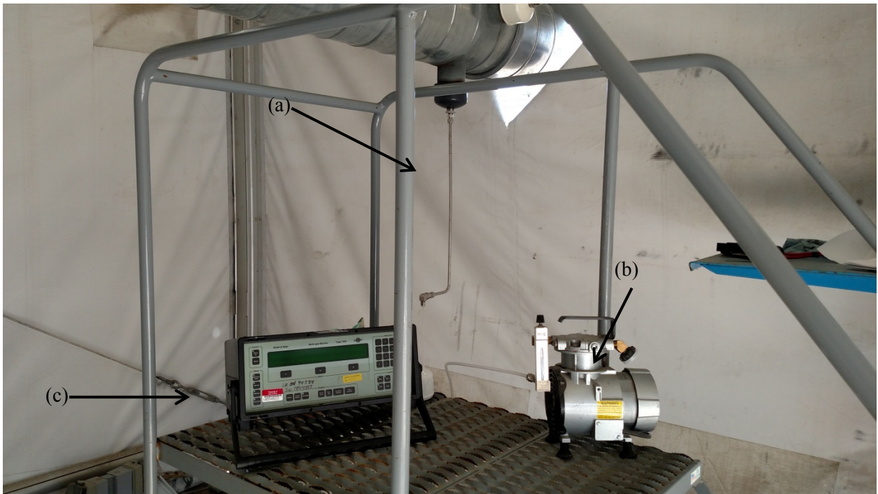
Figure 3.6. Equipment Used for the Gaseous Tracer Sampling: (a) Sampling Probe Installed in a Port, (b) Sampling Pump, and (c) Gas Analyzer
