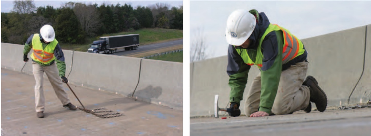
Figure 2.10. Depiction of Chain Dragging (left) and Hammer Sounding (right) on a Bridge Deck (TRB 2013, p. 27)
