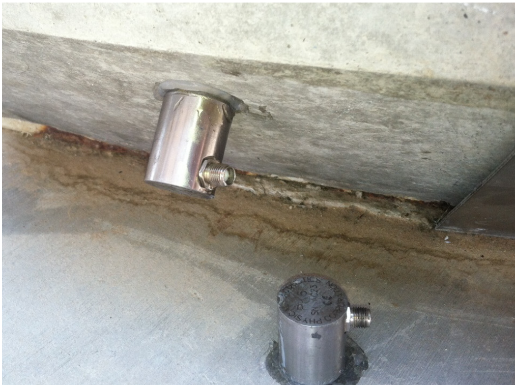
Figure 2.20. Photograph of AE Sensors Bonded to Concrete Surfaces (Courtesy of Paul Ziehl, University of South Carolina)
