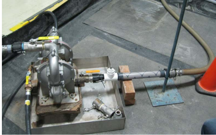
Figure A.15. Static Inline Mixer Detail (to right of pump discharge valve located in center of picture).
