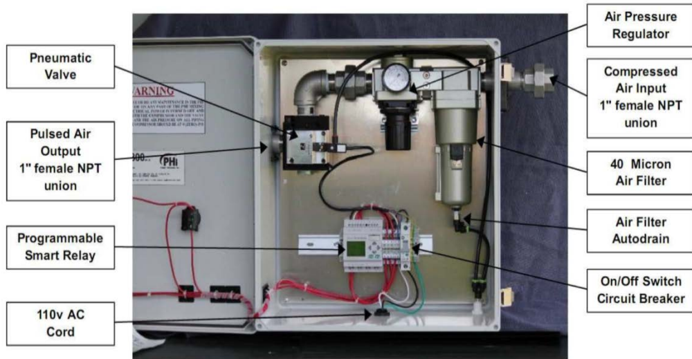
Figure A.81. PHI Mixing System Controller (outside and inside shown).
