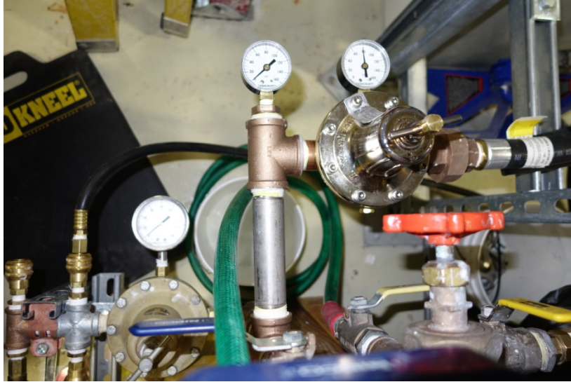
Figure A.27. APEL Room 184 Building Air Regulator and Pressure Gauge.
