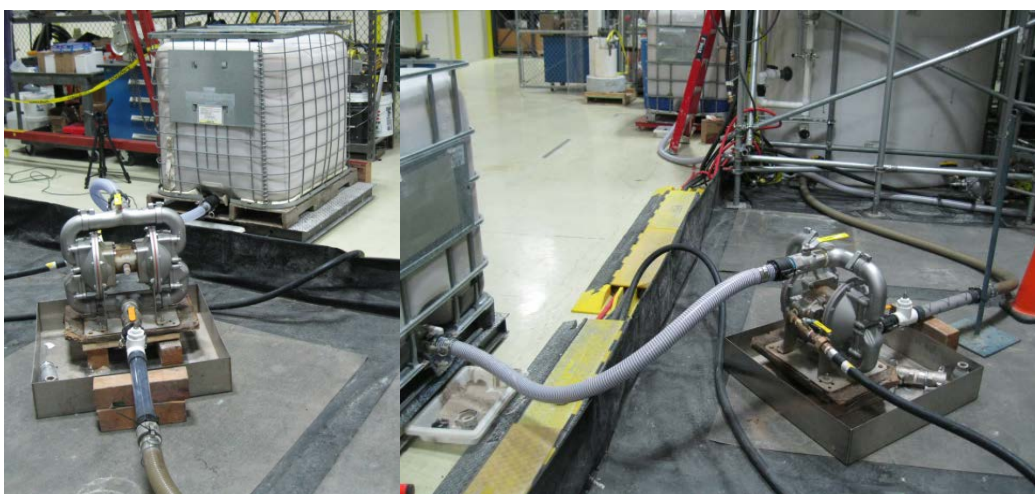
Figure A.14. Clay Slurry Tote and Diaphragm Pump Configuration.
