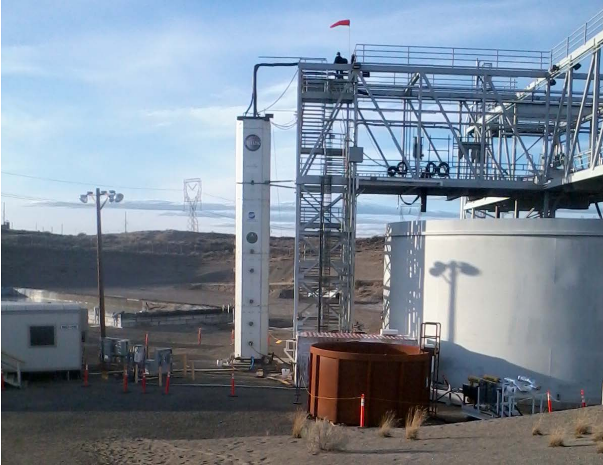
Figure 6.1. Installation Location of the Tall Column at the CTF
