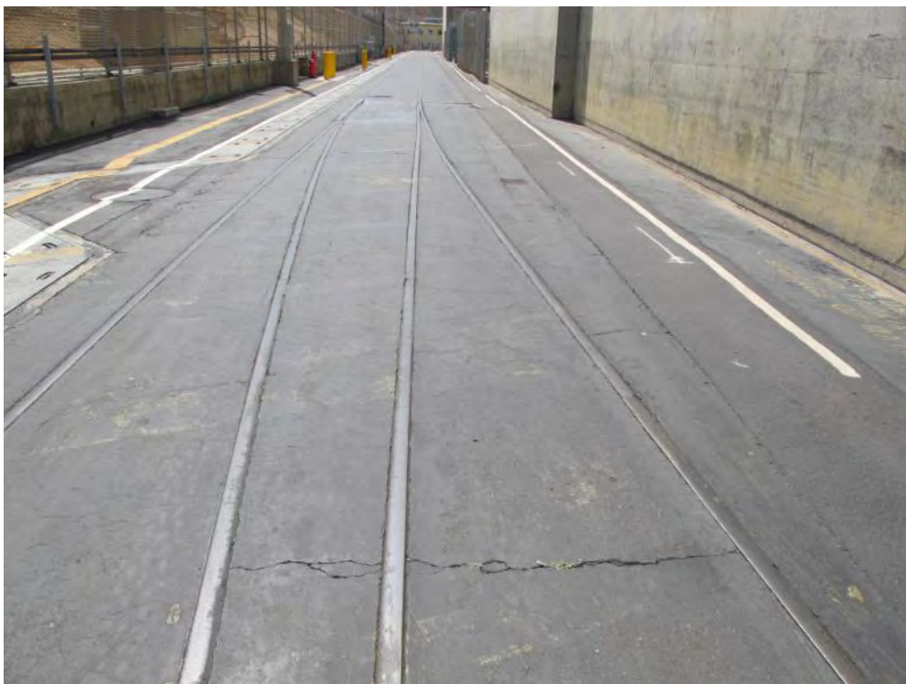
Figure 2-273. Onsite Rail System at San Onofre Site (2015)
