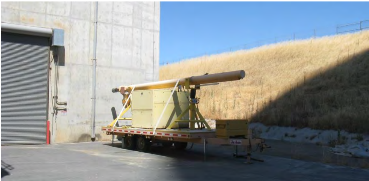
Figure 2-82. Hydraulic Ram Used to Emplace and Withdraw Canisters from Horizontal Storage Modules at Rancho Seco (2013)
