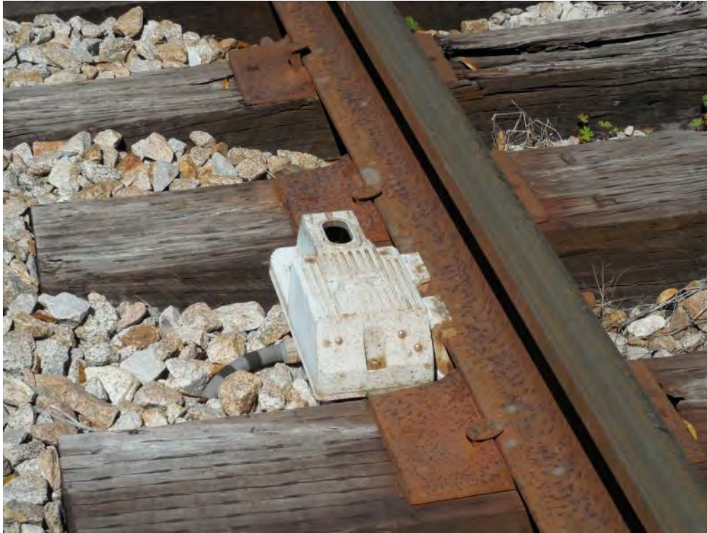
Figure 2-168. Hot Bearing Detector on Florida Northern Railroad (2015)
