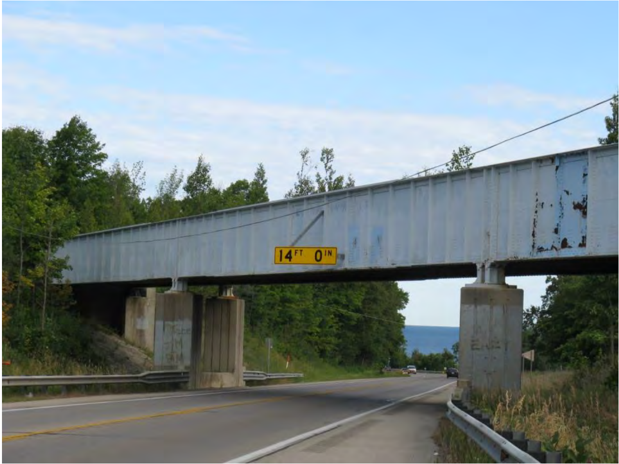
Figure 2-71. Low Overhead Clearance Abandoned Railroad Bridge on U.S. 31 (2013)
