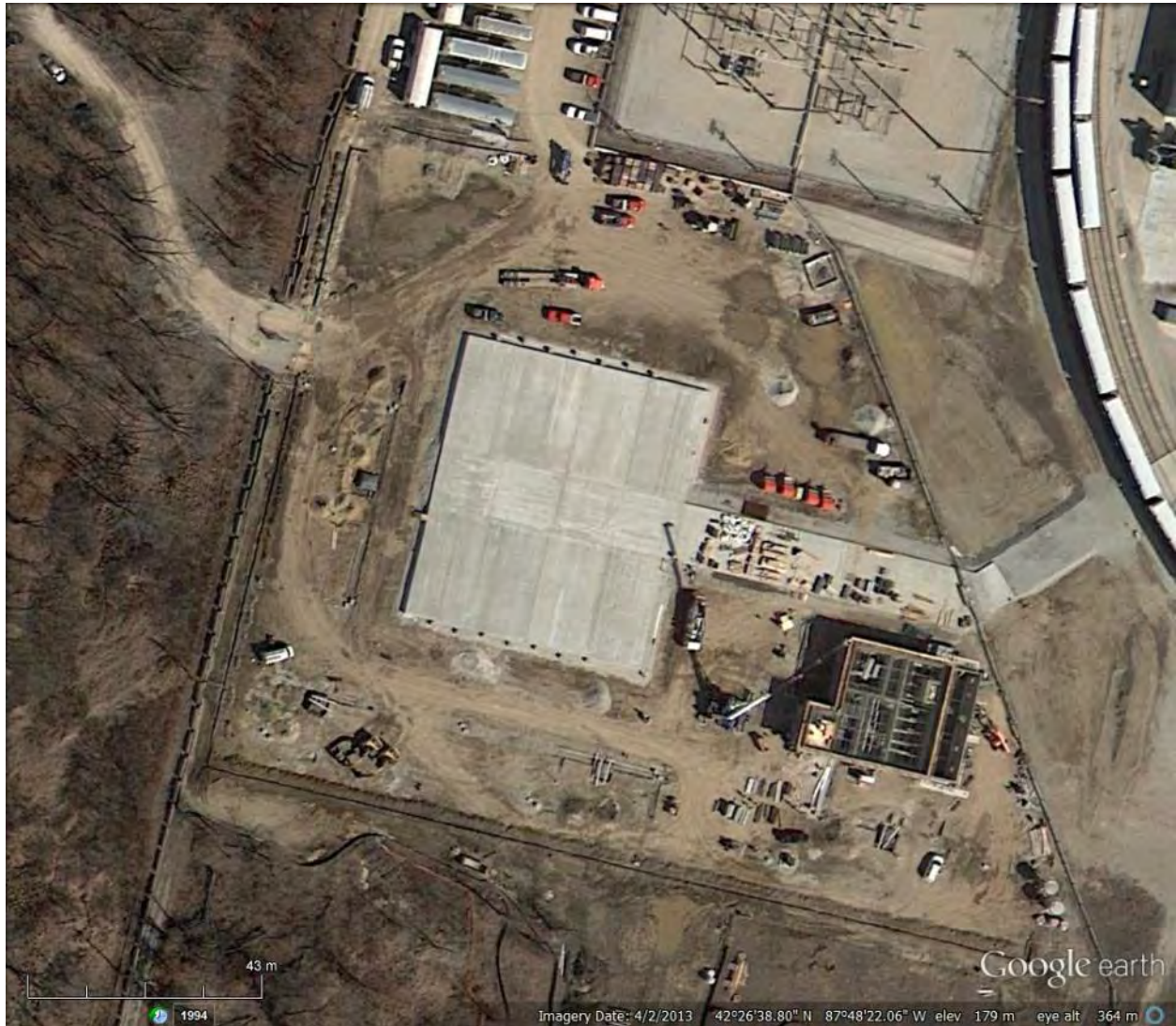
Figure 2-133. Aerial View of Zion Independent Spent Fuel Storage Installation Under Construction (Google 2015)
