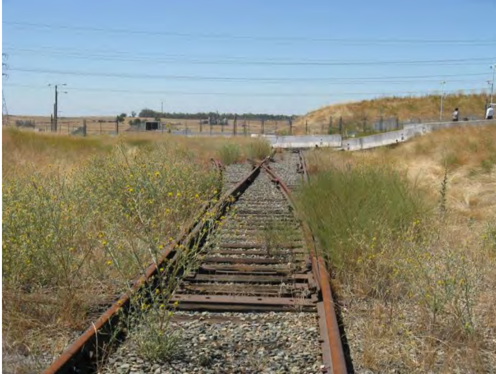
Figure 2-87. Junction of the On-site Track Spur Running Adjacent to the Independent Spent Fuel Storage Installation (Right) and the Longer Track Running into the Rancho Seco Site (Left) (2013)
