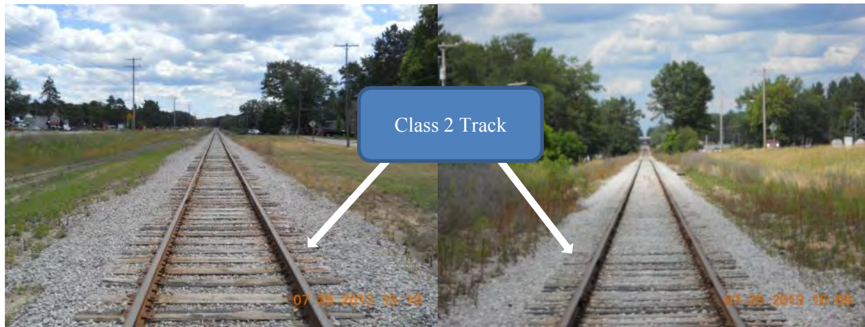
Figure B-9. Track Condition in the Vicinity of Gaylord Transload Location (Looking South) (2013)
