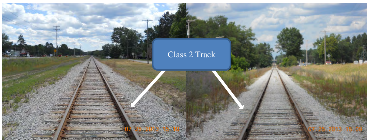
Figure B-9. Track Condition in the Vicinity of Gaylord Transload Location (South)
