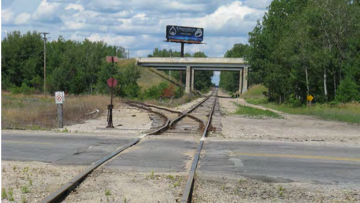
Figure 2-72. Condition of Rail Crossing in 2013 Used for Big Rock Point Reactor Pressure Vessel Transload (Looking North)
