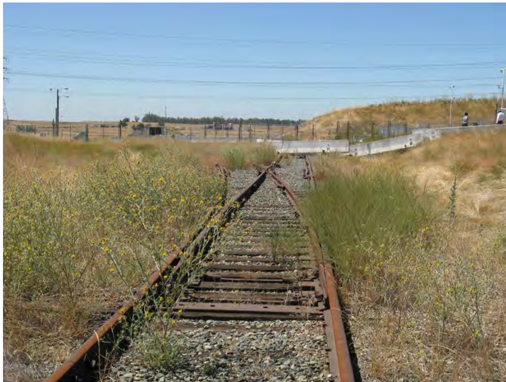
Figure 2-85. Junction of the On-site Track Spur Running Adjacent to the ISFSI (Right) and the Longer Track Running into the Rancho Seco Site (Left)
