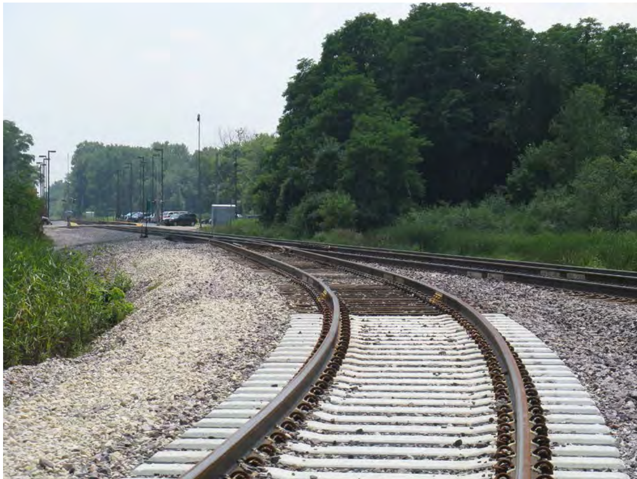
Figure 2-129. Junction of Zion On-site Rail Spur with Union Pacific Railroad Showing Concrete Rail Ties
