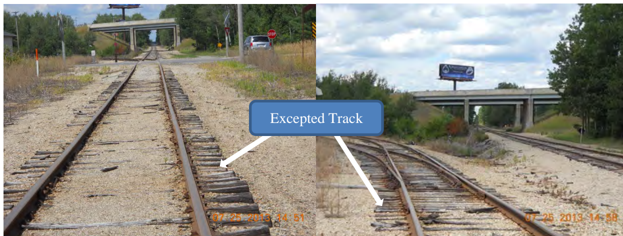
Figure B-8. Track Condition in the Vicinity of Gaylord Transload Location (North)
