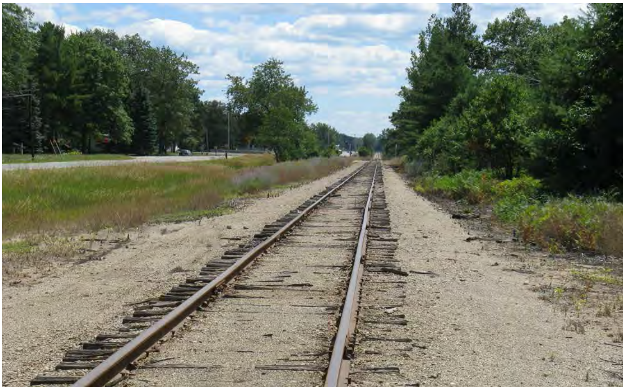
Figure 2-73. Condition of Rail Crossing in 2013 Used for Big Rock Point Reactor Pressure Vessel Transload (Looking South)
