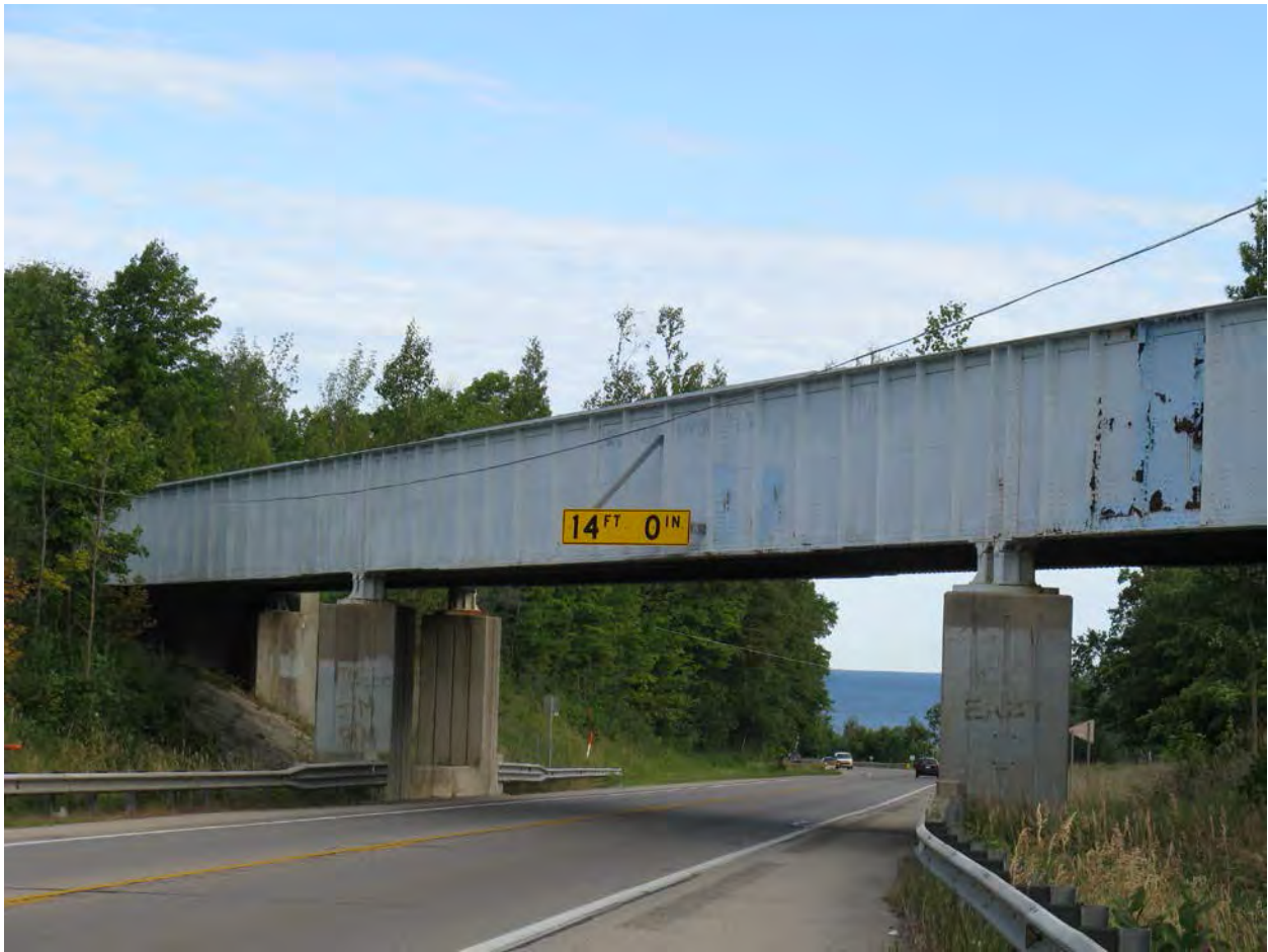
Figure 2-70. Low Overhead Clearance Abandoned Railroad Bridge on U.S. 31
