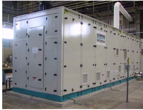
Figure 2: Siemens-Westinghouse SOFC combined heat and power system [3]
