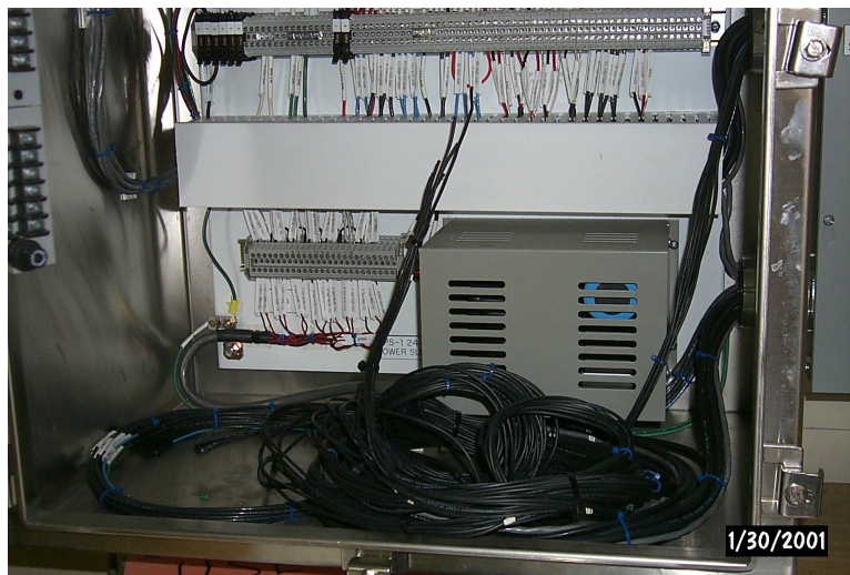
Figure 8.5 Densimeter cables inside panel in DACS trailer
