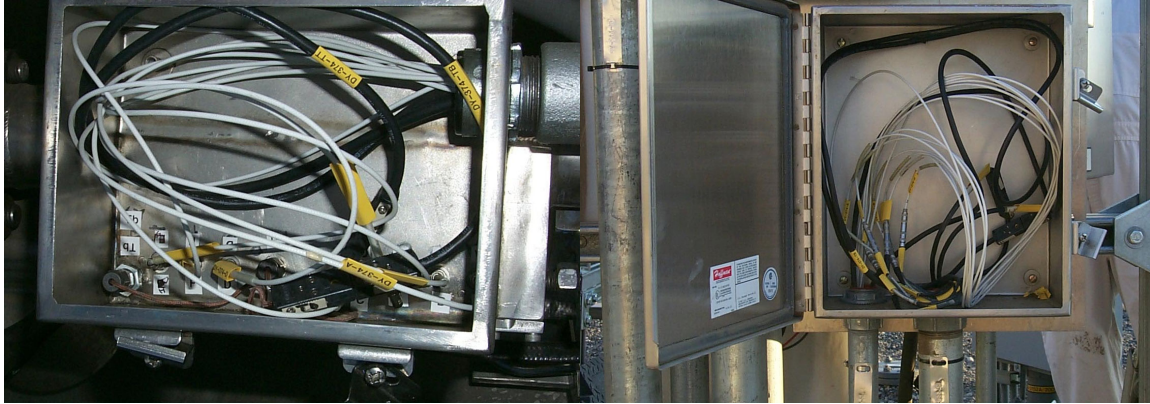
Figure 8.4 Densimeter cable field connections in PPP (left) and junction box (right)
