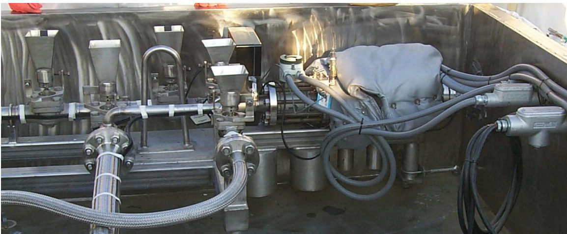
Figure 2.1 Density sensor installed at Hanford in the SY-101 site in the pump pit before and after installation of blanket insulation
