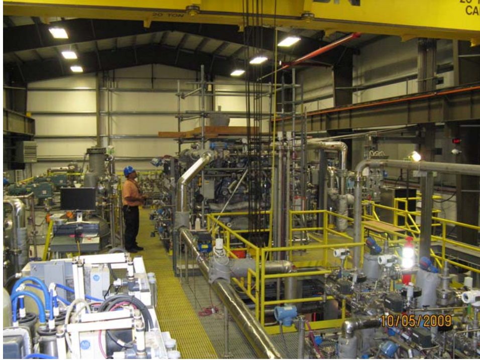
Figure 4.5. Looking South on the Second Floor of the PEP. Readings are being collected from instruments on the upper portion of Tank T02A.
