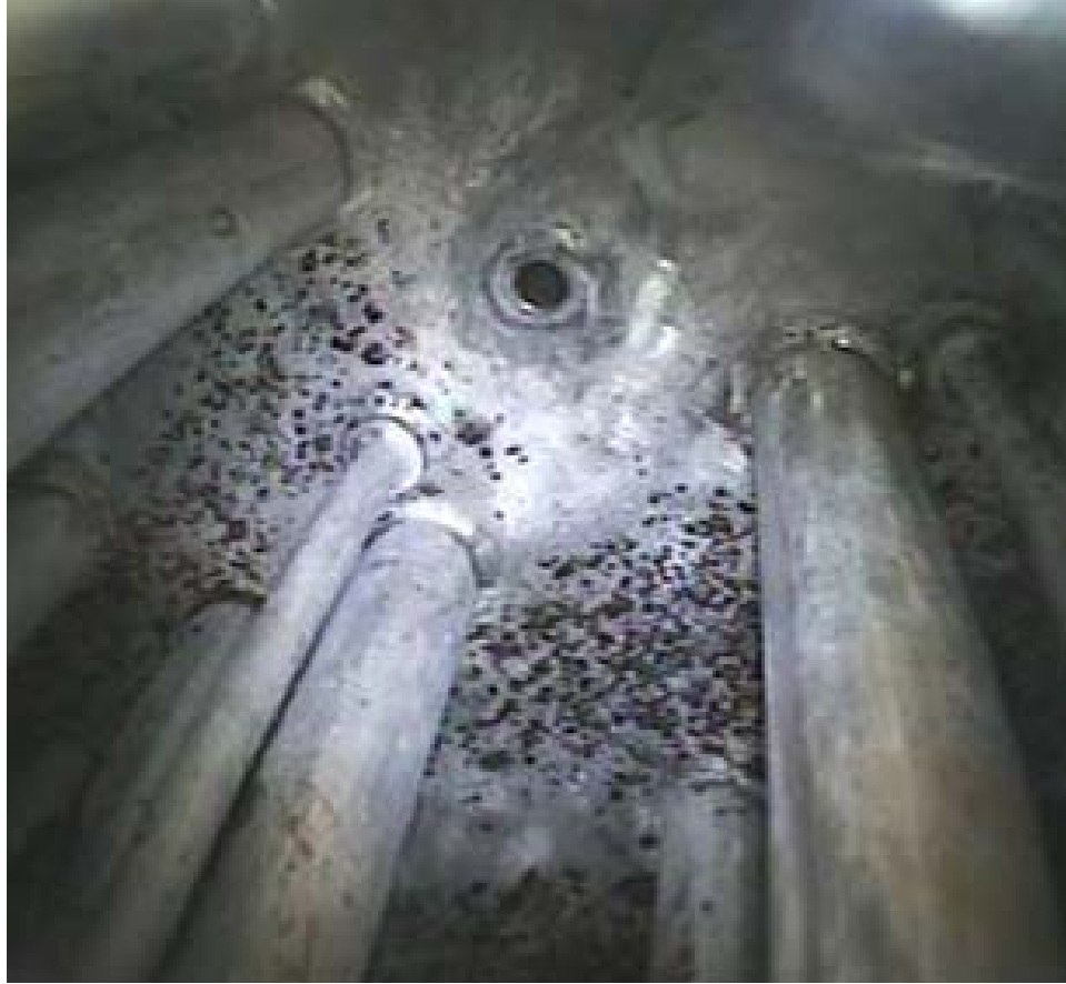
Figure 13.8. Tank T02A After the Prototypic Nitric Acid Cleaning. This is the portion of the tank that was above the acid during the cleaning process.
