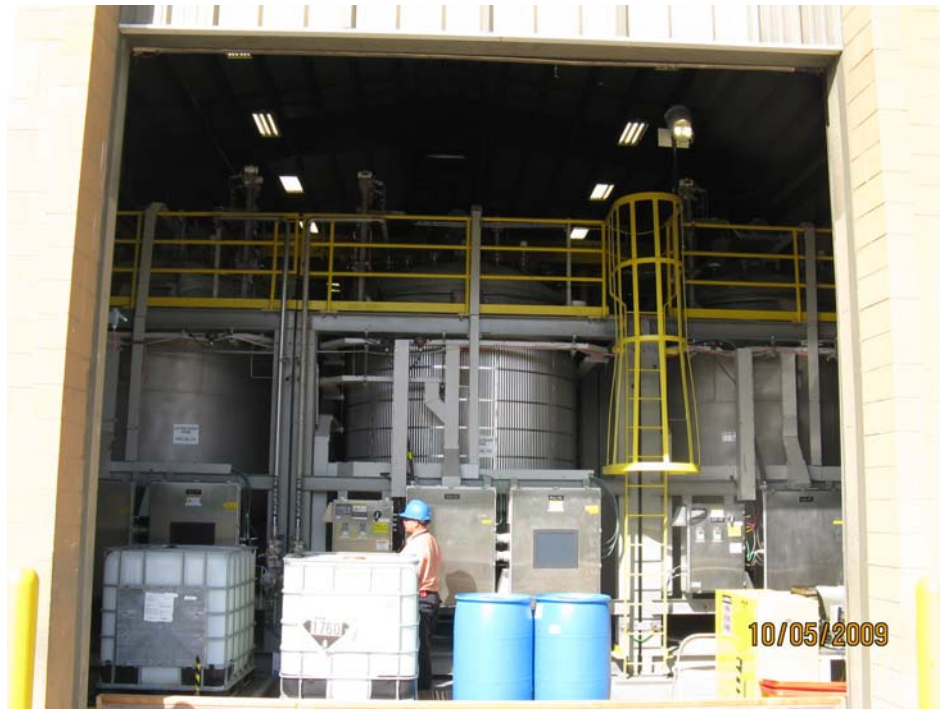
Figure 4.3. Vessels FRP-VSL-T01, HLP-VSL-T22, and FEP-VSL-T01 at Ground Level (looking North)
