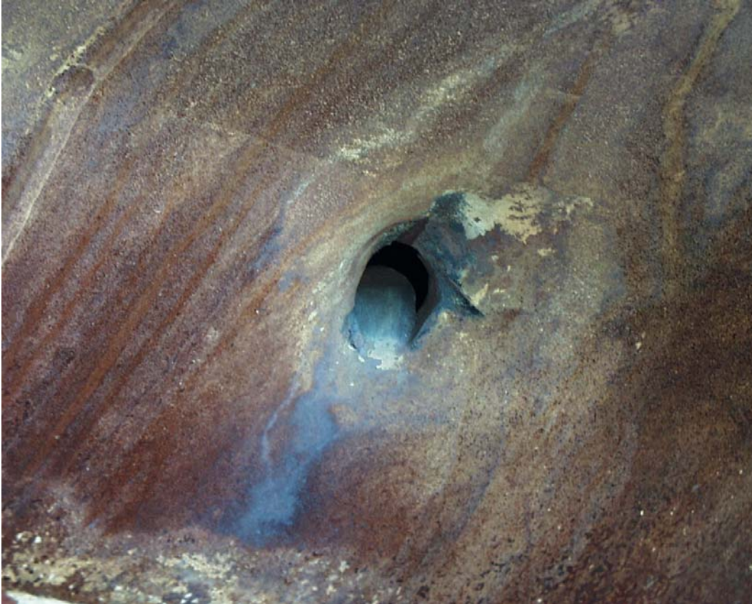
Figure 1.3. Puncture in Tank Car
