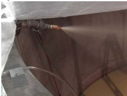
Plugged nozzle at end of cycle 4
