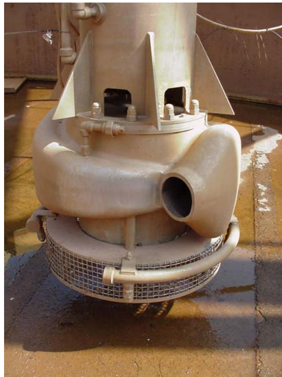
Figure 2.3. Lower Portion of Full-Scale ADMP Installed in the SRS Test Facility (nozzle orientation of mockup ADMP is reversed from full-scale ADMP in Figure 2.2)
