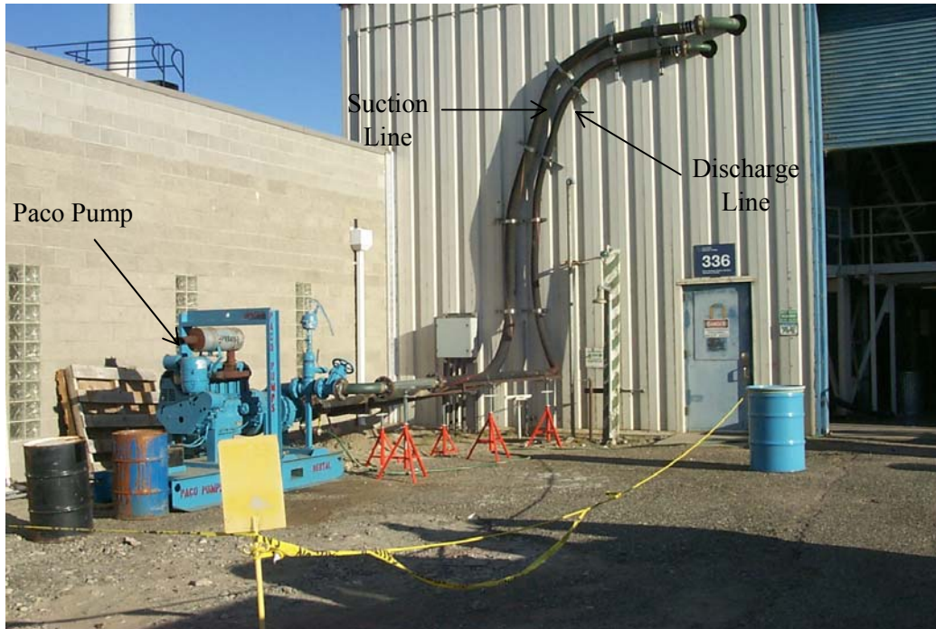
Figure 2.5. Paco Pump Skid Installed Outside the 336 Building Test Facility
