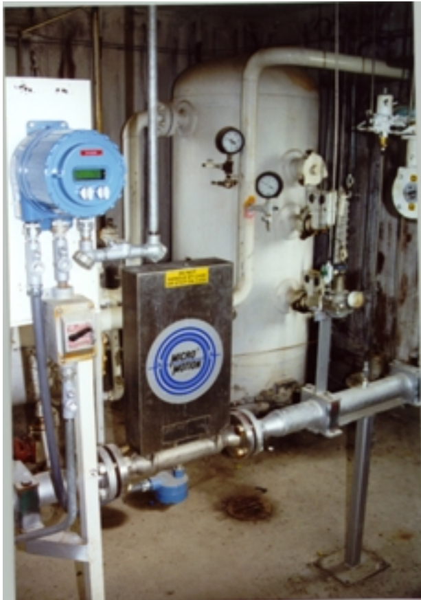
Figure 2. DS150S installed in one of the blue "sheds"
