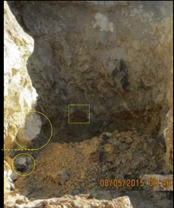
Wooden debris embedded in plug
