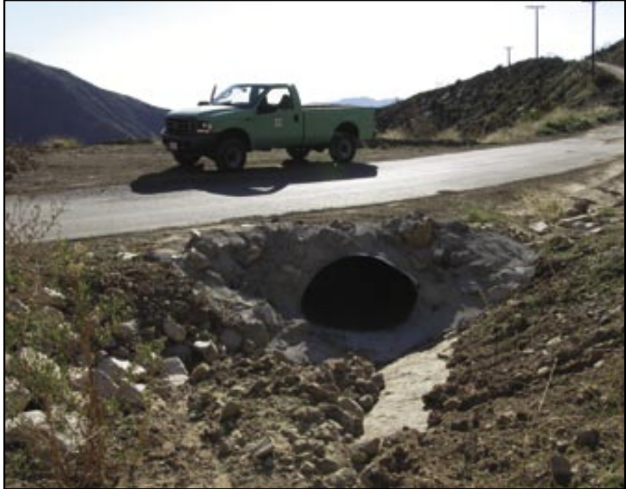
Figure 79—This larger pipe was installed to replace an undersized culvert that had failed in the past.
