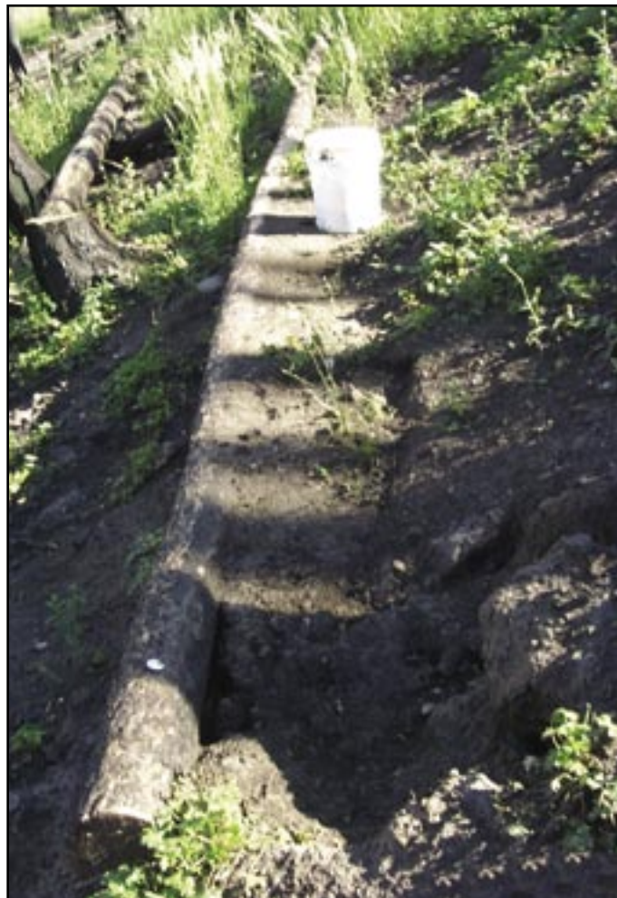
Figure 26—Contour felled LEB which has filled with sediment and then failed. Sediment trapping ability of LEBs on steep slopes is limited.
