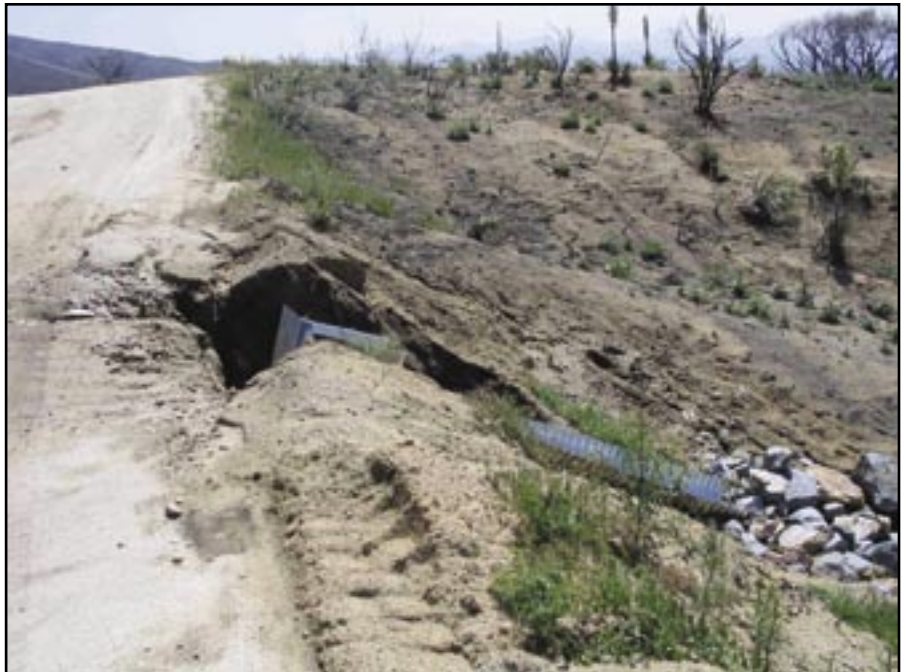
Figure 71—Failed metal roadside drain.
