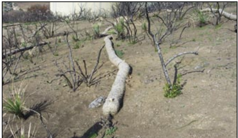
Figure 31—To ensure proper installation, work with experienced crews and inspect as the fiber rolls are installed. Improper installation negates the effectiveness of this treatment.
