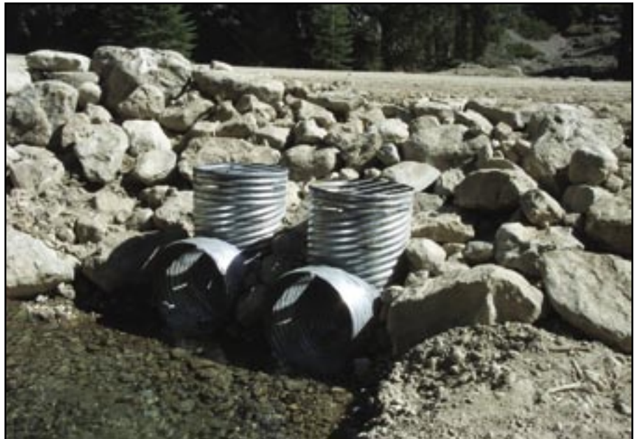
Figure 80—This culvert was modified with two culverts and risers to handle increased flows and potential woody debris.
