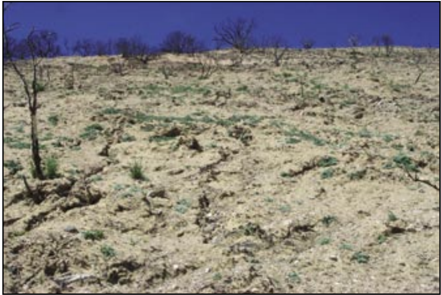
Figure 8—Treated cutslope with rilling. Longer slope lengths tend to have rilling as the runoff concentrates on the surface.
