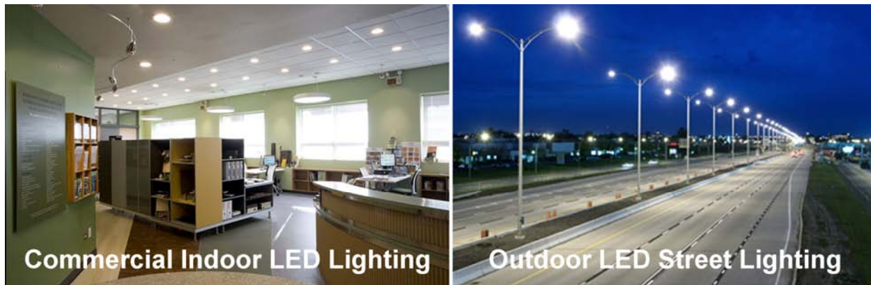
Figure 8-3 (Left) The Chicago Center for Green Technology uses indoor LED lighting to reduce its energy demand for lighting by 64%, freeing the building’s solar panels to produce electricity for other uses. Source: Eric Taub, New York Times, 2/29/2009. (Right) With superior color quality and lifetime and high lumen output, LEDs are the emerging technology for the next generation of outdoor lighting. Source: Luminus Devices, Inc.
