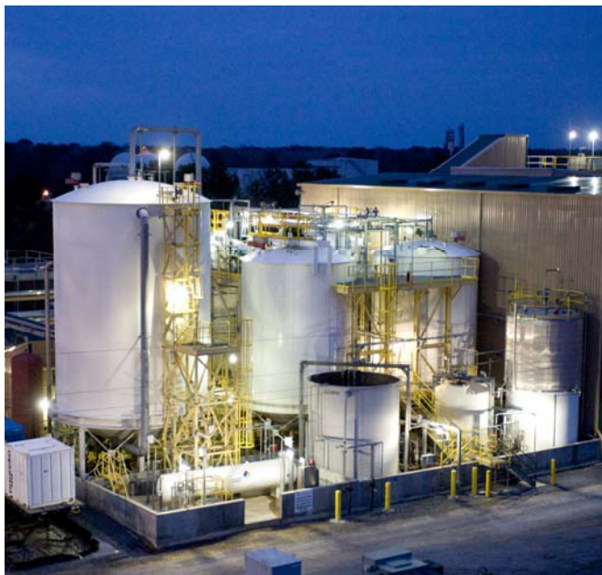
Figure 9-4 Second-generation cellulosic biofuel demonstration facility. Source: Verenum Corp.
