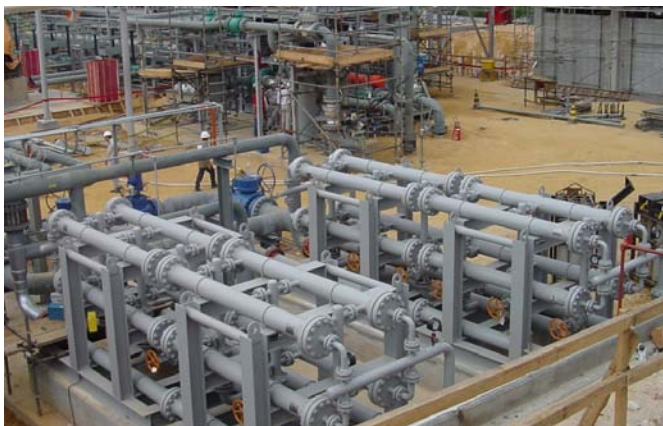
Figure 18. A membrane plant for natural gas processing (courtesy MTR, Inc.).
