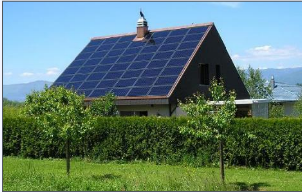
Solar Photovoltaic (PV)
