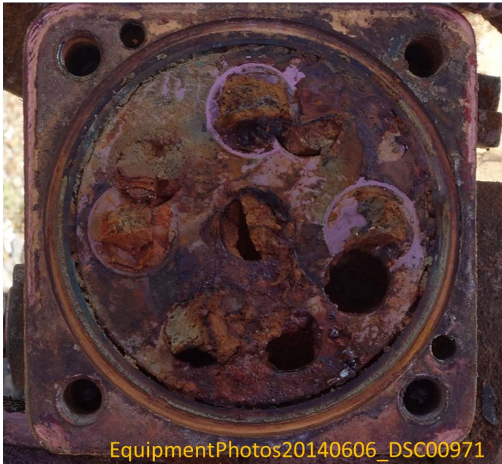
Figure 6.7 – Photograph of "Pipe Rams" Selector Valve Rotor taken during Inspection
