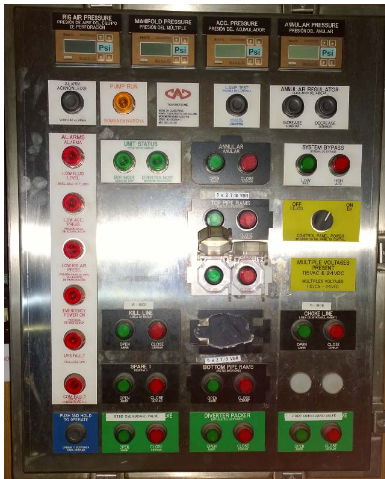
Figure 3.8 – Photograph of Remote Well Control Panel in Toolpusher's Office
