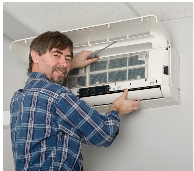
Ductless heat pump systems use 30 to 50 percent less energy to heat homes than electric-resistance or forced-air systems.
