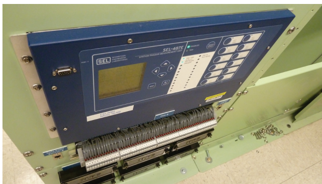
BPA has installed 126 phasor measurement units at 50 key substations and large wind generation sites throughout the Northwest. These shoe-box sized devices transmit precise power system data 60 times a second, giving operators a wide-area view of the system.
