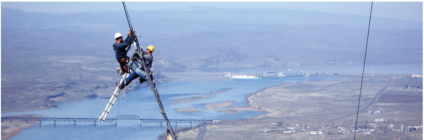
BPA linemen install a helical connector shunt on the Midway-Vantage 230-kV line in central Washington, north of Hanford.
