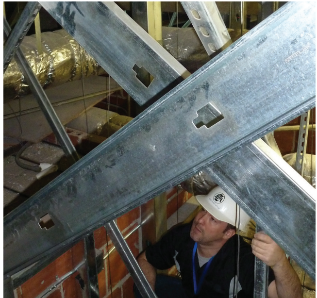
BPA installs steel braces at facilities to make them less vulnerable to a major earthquake.
