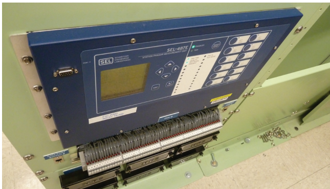
BPA has installed 126 phasor measurement units at 50 key substations and large wind generation sites throughout the Northwest. These shoe-box sized devices transmit precise power system data 60 times a second, giving operators a wide-area view of the system.
