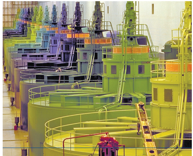
Hydroelectric generators turn the power of the Columbia into energy for Northwest homes and businesses.
