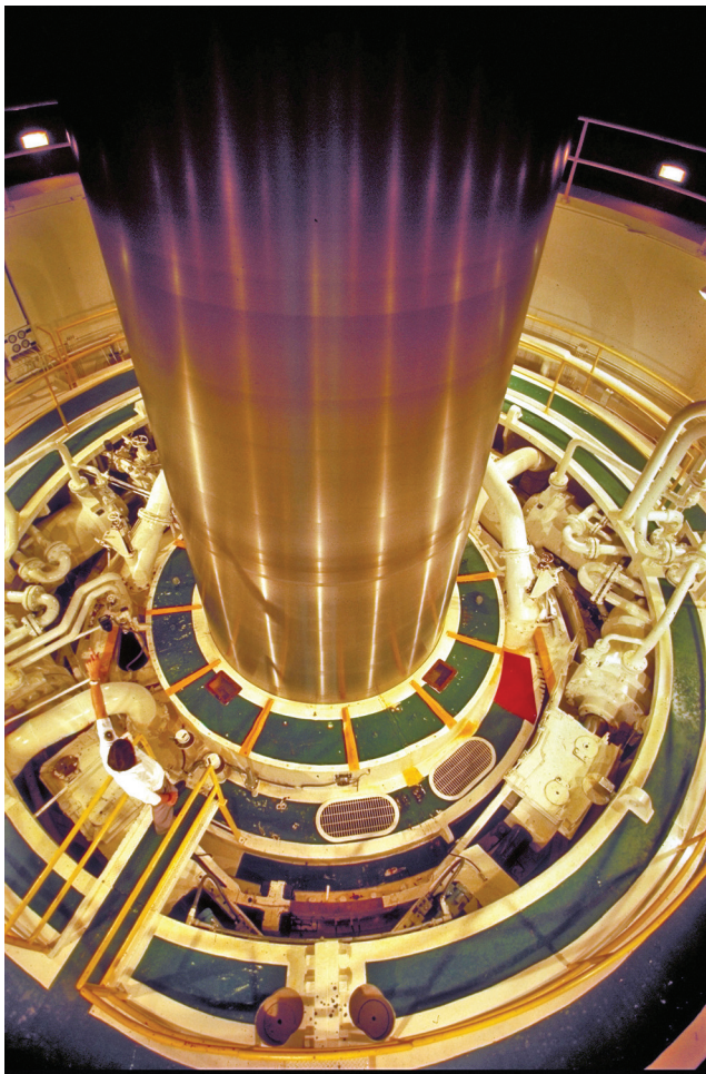
A turbine shaft spins at Grand Coulee Dam.
