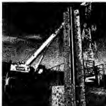
The cruciform shape of this tower footing is saving BPA millions. It's easier and cheaper to manufacture than the original design.
