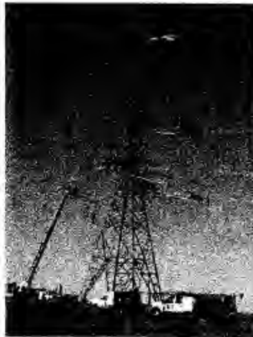
A helicopter hoists platforms for linemen during the construction of this single-circuit 500-kilovolt tower – one of hundreds on the McNary-John Day line saving BPA big bucks.
