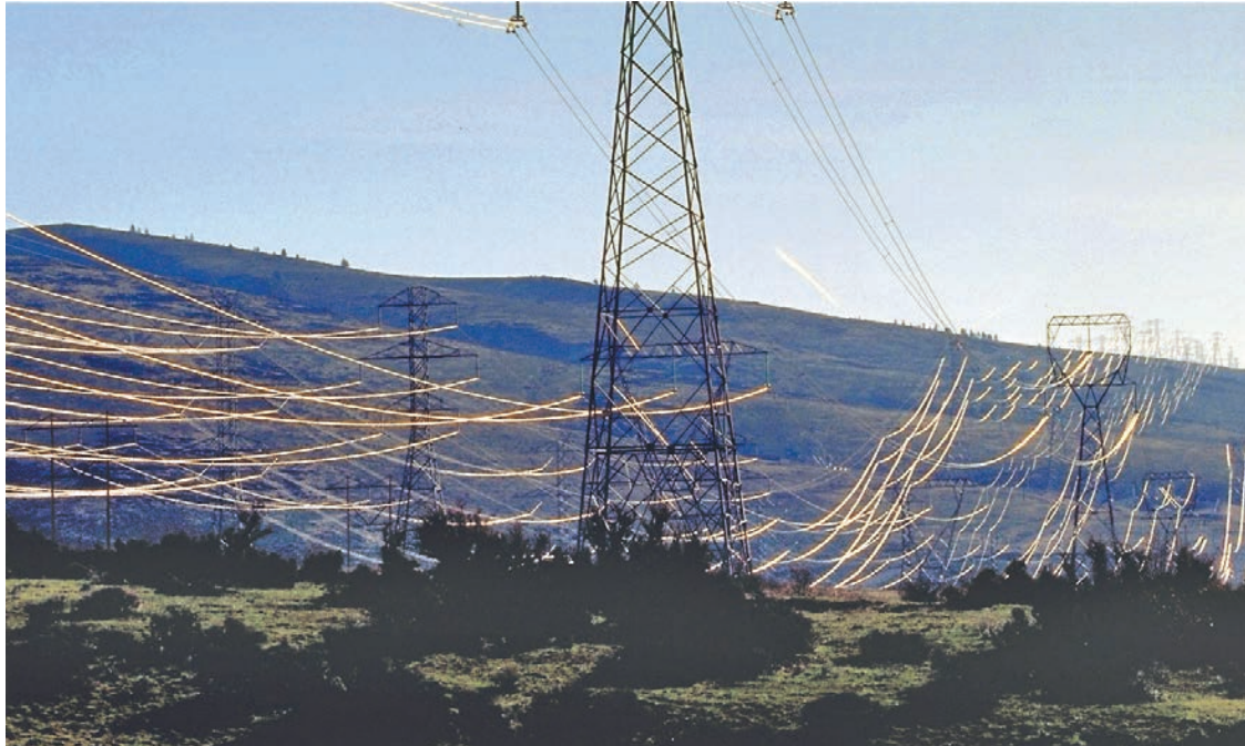
Transmission lines connected to BPA's Schultz Substation near Ellensburg, Wash., helped BPA avoid stretching a new line across the Cascades.
