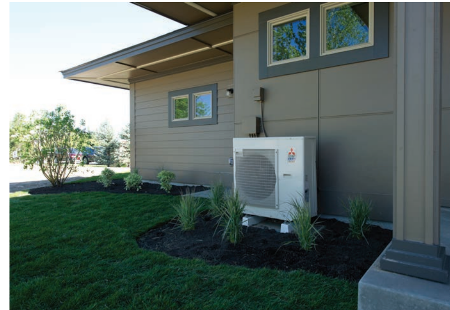
Ductless heat pumps (such as the outdoor compressor unit shown here) proved to offer significant energy savings for single-family homes when NEAA field tested them in 2006 to 2008. BPA was a major contributor to their success. In 2011, tests were under way to evaluate ductless heat pumps for use in manufactured homes, multifamily homes and small commercial buildings.
