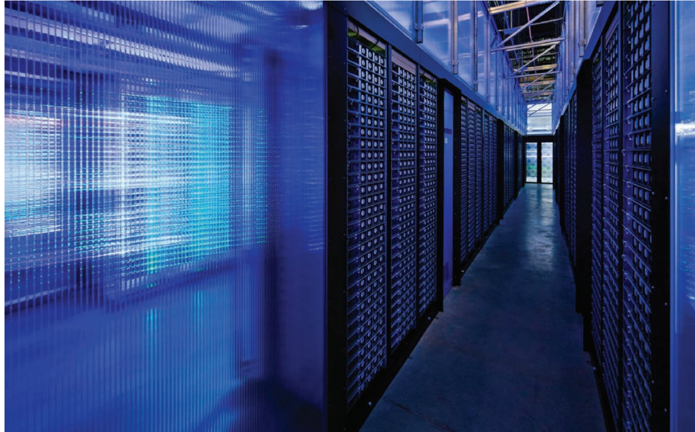
The efficient design of Facebook’s data center in Prineville, Ore., reduces energy consumption. BPA’s transmission system helps supply the data center with electricity. (Facebook)
