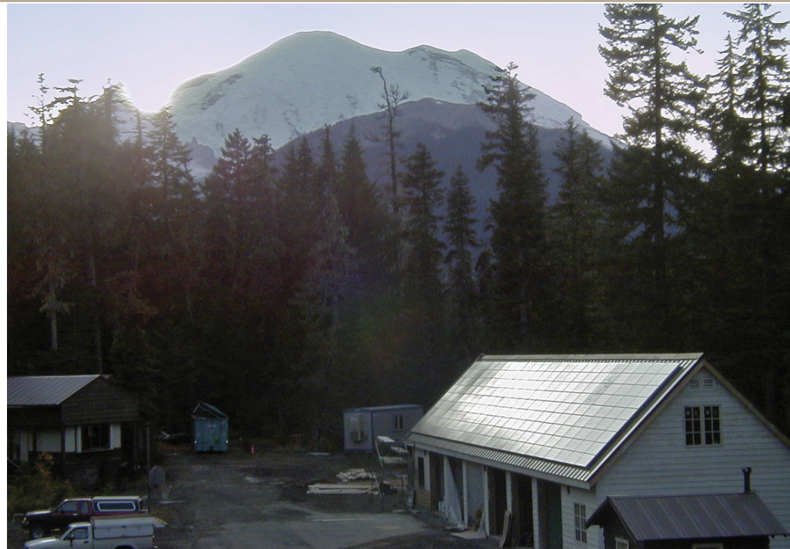
This 20-kilowatt photovoltaic installation was contracted by BPA engineers on a service building at Mt. Rainier National Park; it operates off the transmission grid, dramatically reducing the use of a diesel generator.
