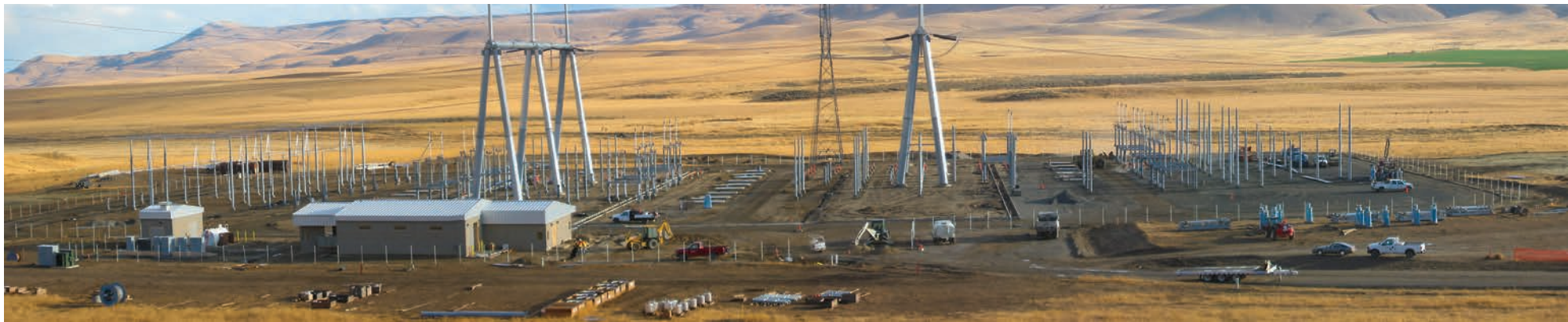
Wautoma Substation, the southern end of the Schultz-Wautoma transmission line in Washington.
