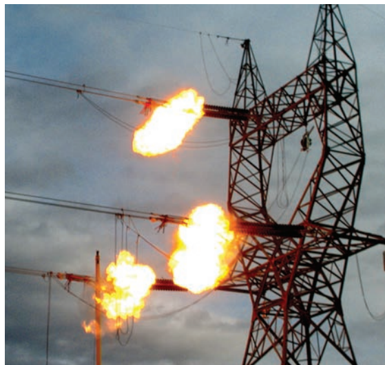
BPA used implosive fittings during construction of its Grand Coulee-Bell line. The fittings employ explosives to compress a metal sleeve around the end of the conductor, locking it into place.
