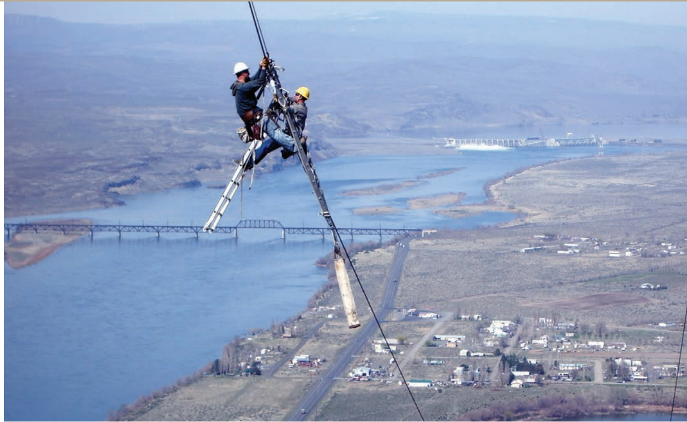
Far above the Columbia River, linemen install splice shunts on BPA's 230-kilovolt Midway-Vantage line. The shunts strengthen lines without taking them out of service, saving ratepayers millions of dollars. (Barry Peckham/BPA)
