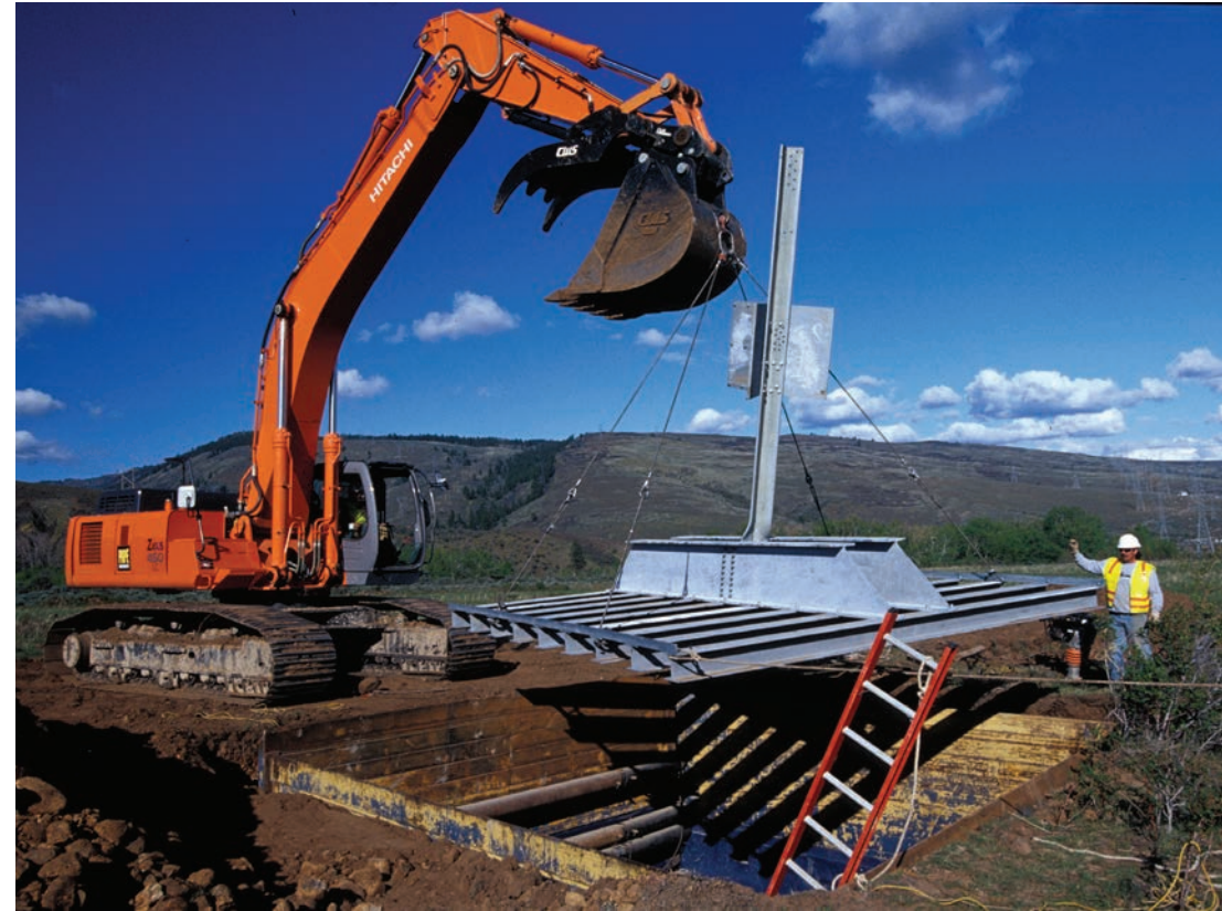
Crews install a transmission tower footing during construction of BPA's Schultz-Wautoma line.
