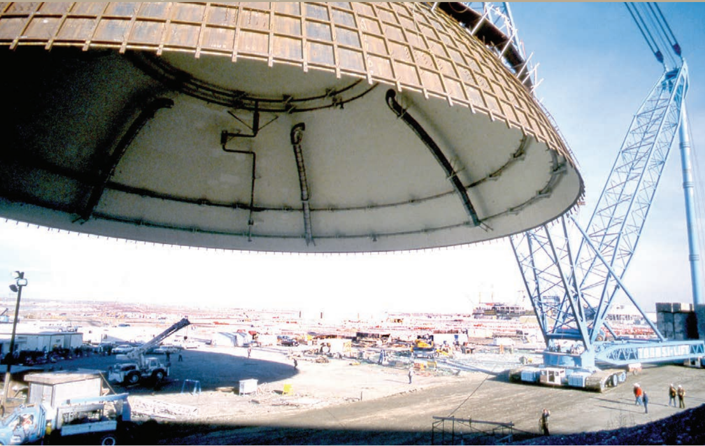
Work begins on Washington Nuclear Plant 1, developed by the Washington Public Power Supply System with financial backing from BPA.
