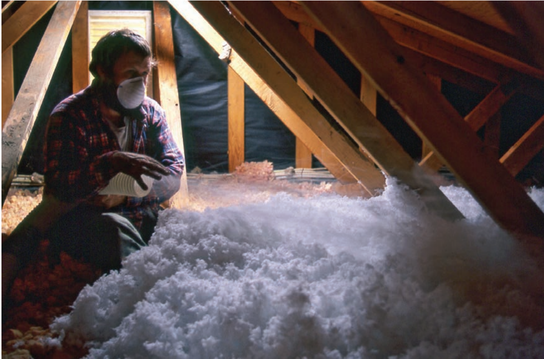
Home weatherization was a flagship of the first suite of BPA conservation programs. Contractors retrofitted insulation in the attics, walls and crawlspaces of electrically heated homes to reduce their energy usage.
