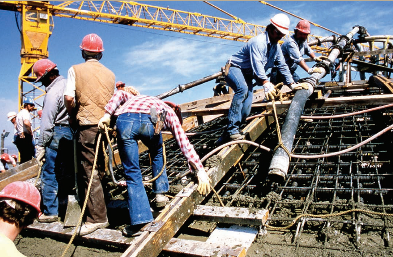
Workers pour concrete for the containment dome at WNP-2. Now known as the Columbia Generating Station, it was the only nuclear plant completed. Energy Northwest (formerly WPPSS) owns and operates the plant and BPA purchases and markets its output.
