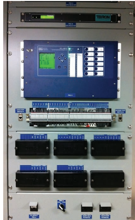
More than 100 phasor measurement units, or PMUs, monitor BPA’s transmission system.
