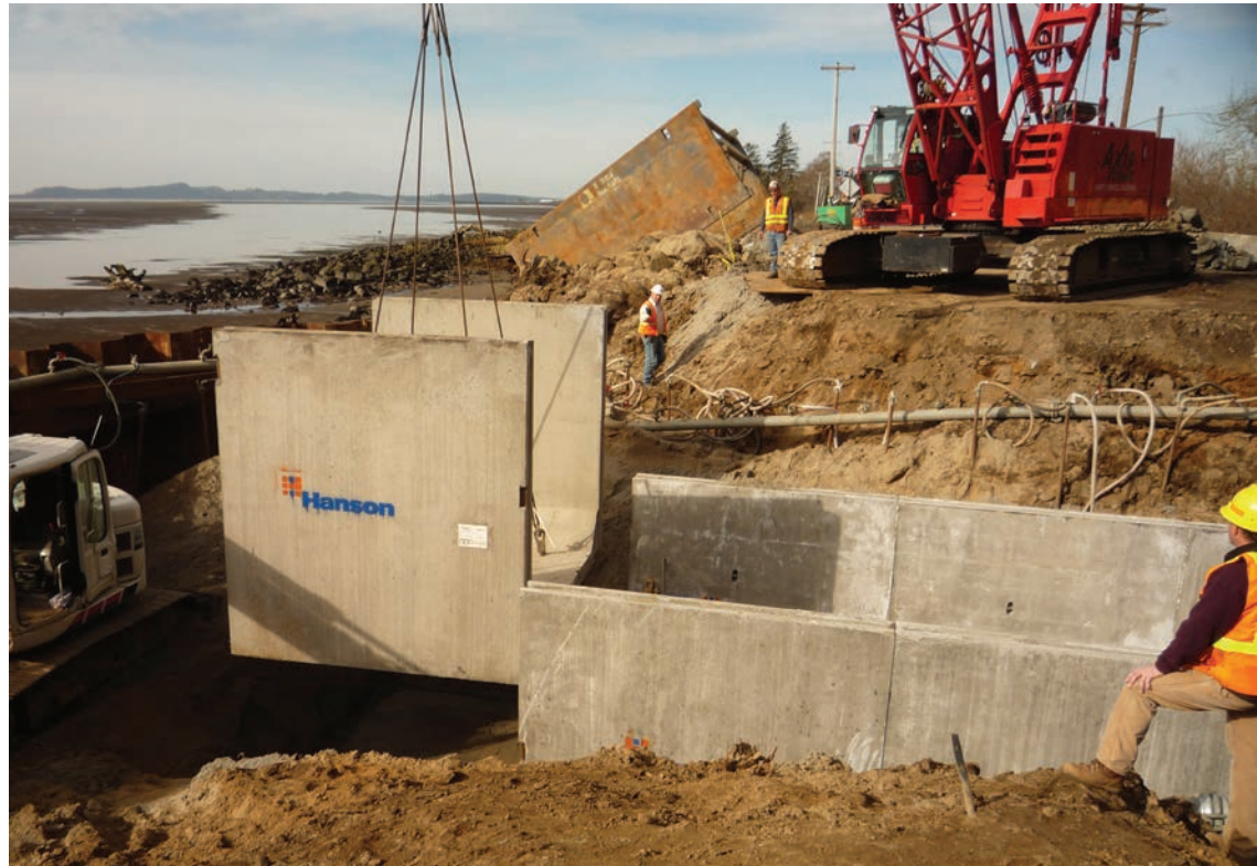
Workers install a large culvert to reopen historic wetlands in the Columbia River estuary to provide food and refuge for juvenile salmon and steelhead. The young fish build strength in the estuary before setting out into the ocean. (David Wilson/BPA)
