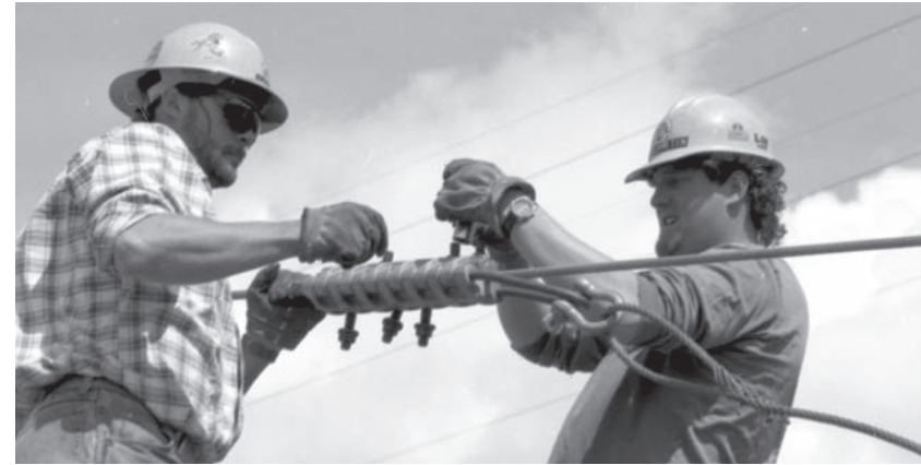
BPA crews have installed thousands of miles of fiber optic cable on existing transmission towers.
