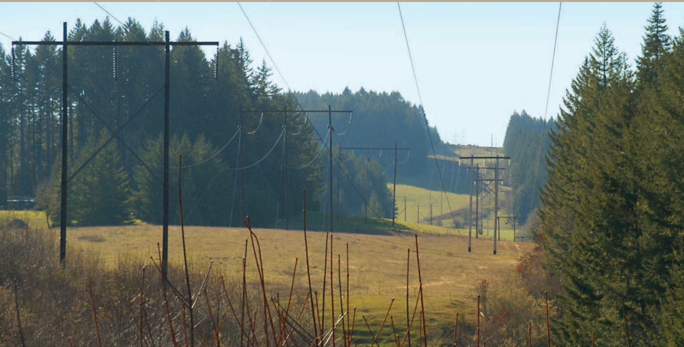
BPA replaced the wood poles on its Albany-Burnt Woods and Santiam-Toledo transmission lines in the summer of 2009. Vegetation stands well back from the lines.
