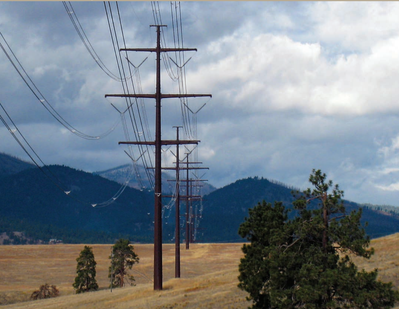
Residents selected the single-pole tower design for its reduced visual impact.
