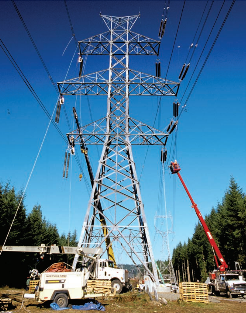
Double-circuit towers that support two sets of transmission lines helped reduce the environmental impacts of BPA's Kangley-Echo Lake line. (Lou Driessen/BPA)
