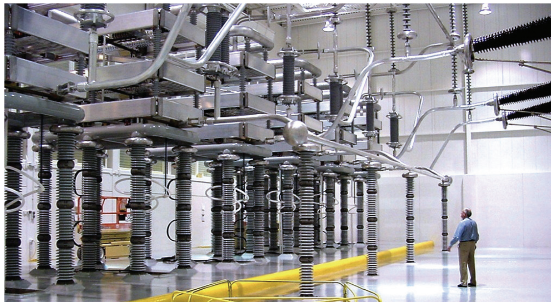
Modernization of BPA's Celilo Converter Station included replacement of decades-old mercury arc valves with solid-state technology to convert alternating-current electricity to direct-current for transmission to Southern California.
