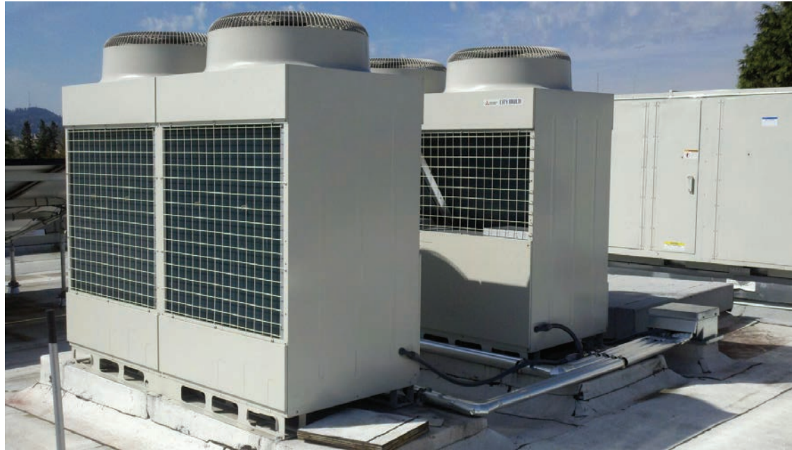
Roof unit, commercial building ductless heat pump.
