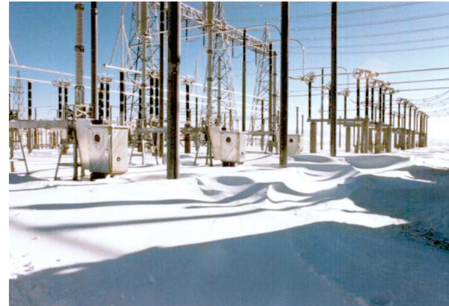
During a Montana cold snap in 1989, equipment at Garrison Substation choked in the sub-zero temperatures.
