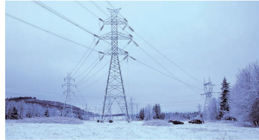
Construction crews didn't know it, but they completed Kangley-Echo Lake just in time to beat a massive 2003 snowstorm. If the line had been energized a few days later, the transmission grid in the area might not have been able to handle the demand.
