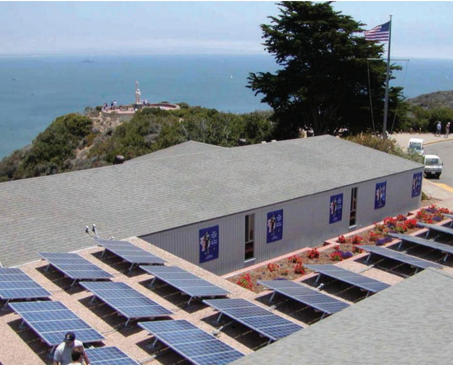
This 10-kilowatt photovoltaic array at Cabrillo National Monument in San Diego, was designed and contracted by BPA engineers under a reimburseable cost agreement with the National Park Service. Beginning in the mid-1990s, BPA contracted out to other public agencies to design and install energy efficiency and renewable energy system projects.
