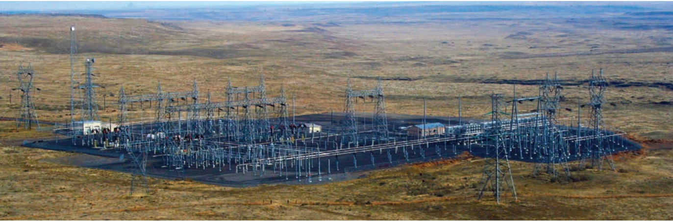
In the heart of the Columbia River Basin's wheat-growing region, BPA's Slatt Substation became home to the world's first 500-kV flexible alternating-current transmission system devices, or FACTS, which control the flow of power on transmission lines.
