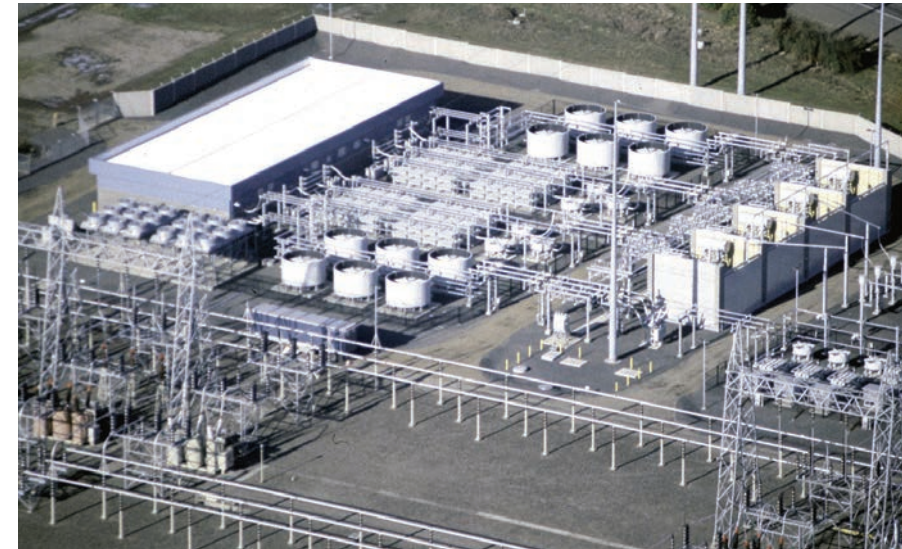
BPA's Keeler Substation (below), near Portland, is home to the fast-acting devices (above) which help stabilize power swings on the system caused by short circuits or other disturbances.
