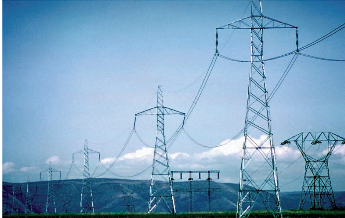
Improvements doubled the capacity of the direct-current intertie, in the foreground, without adding to the wires already in the air.
