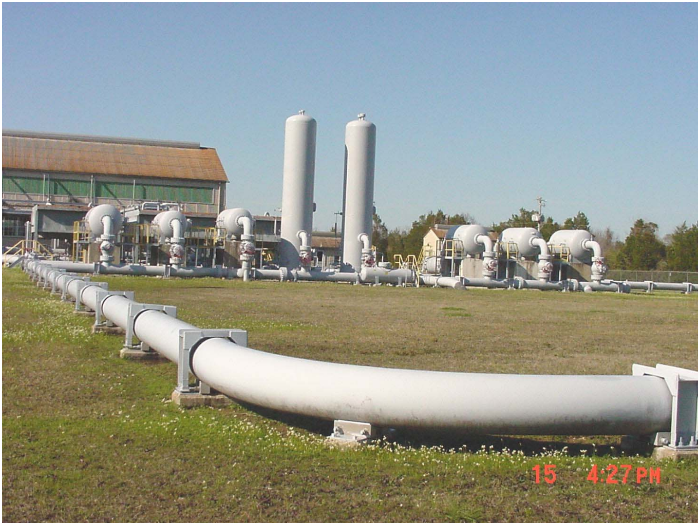
Mainline natural gas pipeline entering the Gallion Compressor station near DeMopolis, Alabama, with a view of the scrubber towers and filter units used to eliminate contaminants prior to compression operations. Courtesy Southern Natural Gas Company, El Paso Corporation.
