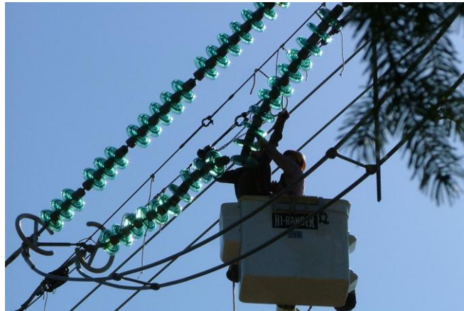
Damaged insulators create a dangerous situation that can result in a power outage and put anyone nearby at risk of electric shock, serious injury or death. (BPA photo)
