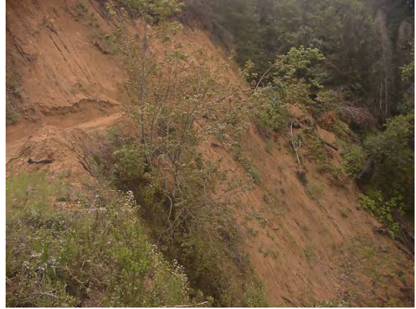
Little Sur River – Road Cut
