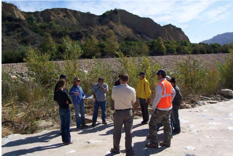
Figure 7. Santa Paula Creek Flood Control Project fish ladder, October 2009. Note fish ladder filled with sediment and growing vegetation (willows and alder).
