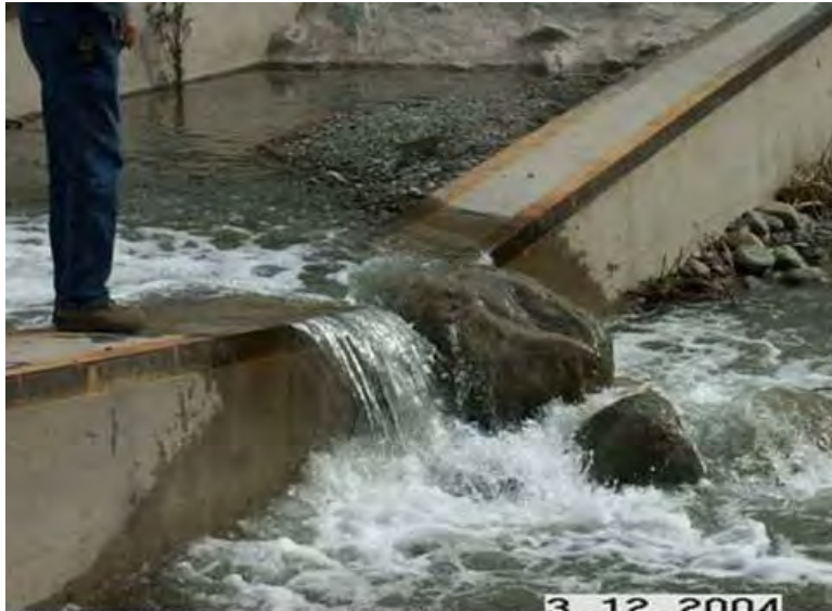
Photo 13. March 12, 2004 – Looking east at fish ladder weir notch obstructed with large boulders.
