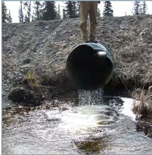
The perched culvert before replacement prevented fish passage.
