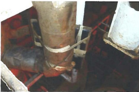
Figure 19: Set up for radiography at HD-P-01-08, 3" elbow (UT not performed due to insulation).
