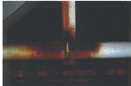
Figure 14: Set-up for radiography of 2" pipe upstream of BDV-V20 (item is not part of annual inspection cycle).
