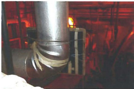
Figure 10: Set up for radiography at HD-P-01-05, 3" elbow (UT not performed due to insulation).
