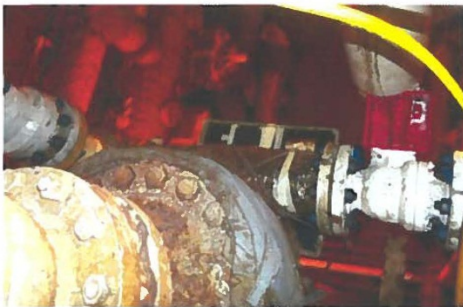
Figure 13: Set up for radiography at HD-P-01-05, 3" pipe (UT not performed due to insulation).
