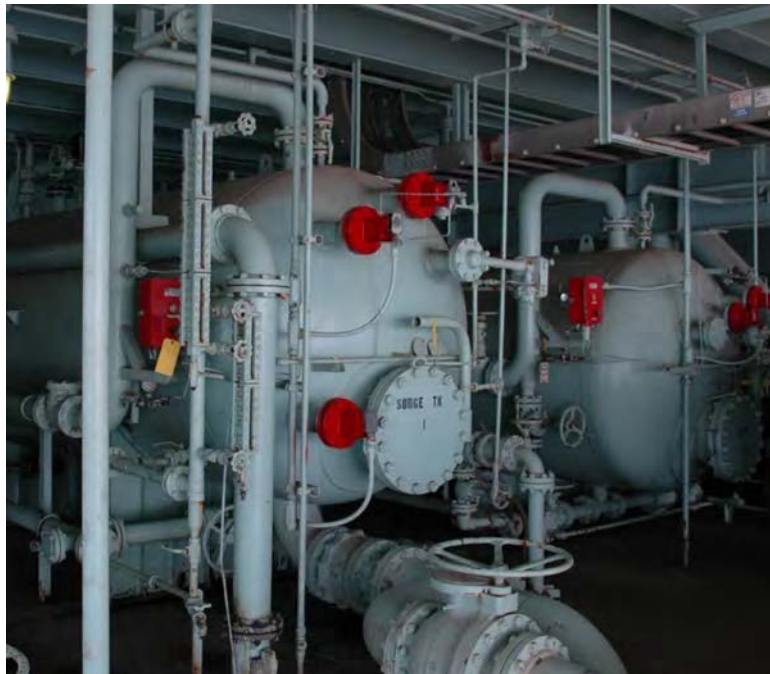
Figure 2 – Surge and CTS (right) Tanks on board Platform Houchin. (BSEE photo)
