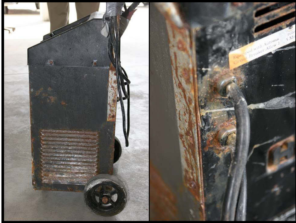
Figure 33: Rig Battery Charger weathering, side and back
