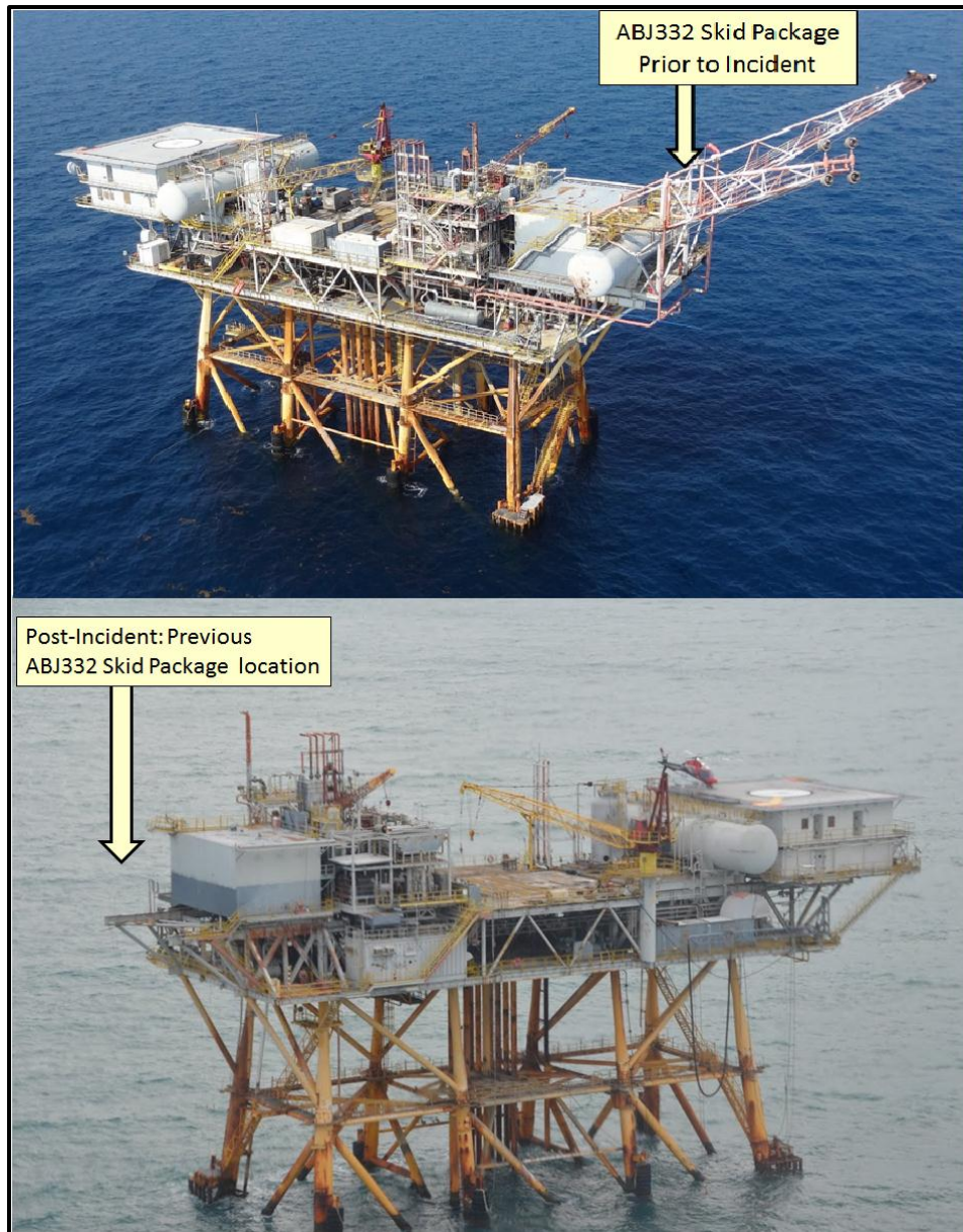
Figure 6: Aerial Before & After Photos of Vermilion Block 200 Platform “A” (Top Photo from Talos/ERT-OFS June 28, 2012 Site Visit; Bottom Photo from Panel Site Visit, November 14, 2013)
