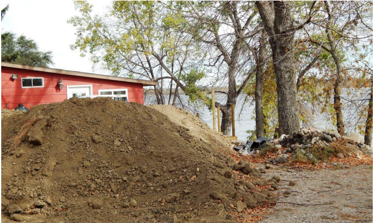
This picture was taken looking northeast from the northern section of Cabin Area A, Jamestown Reservoir. The mounded dirt looks like the beginnings of an addition on to the "cabin". A deck can be seen in the background (not a dock).
