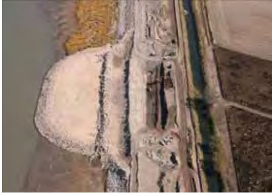
Figure 1 - Contractor repairs the area where seepage was discovered at A.V. Watkins Dam in November 2006 – October 22, 2008
